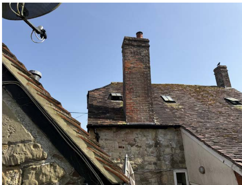
Photo 1: View of the main chimney stack from the rear roof slope, showing brick staining and eroded pointing.
