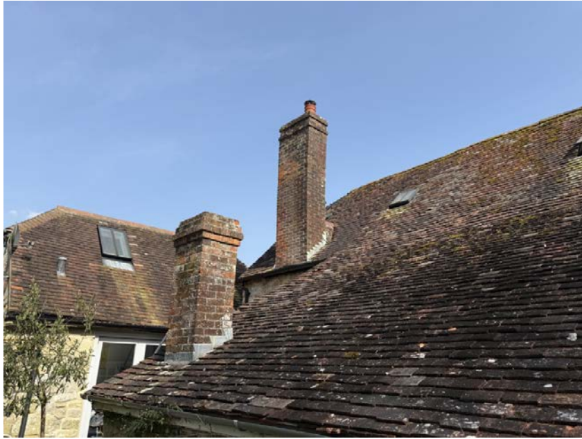
Photo 3: Wider view showing the main leaking stack alongside the smaller stack to the rear of the property Lead flashing is visible at the roof abutment of the nearer, shorter stack; the base of the taller, defective stack slightly obscured and is difficult to inspect from ground level.
