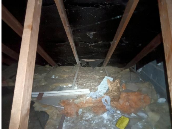
Plate 7. Loft insulation and torn roof lining inside B1 roof void.
