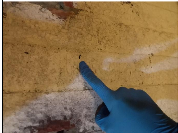
Plate 8. Brown long-eared bat dropping found in roof void.
