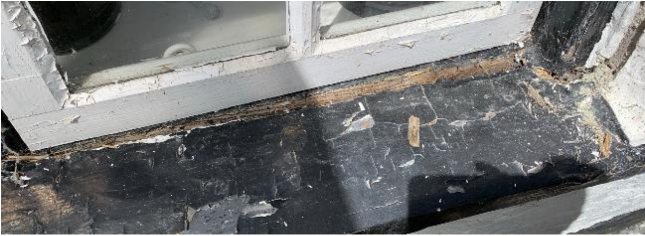
Current state of outside sill split and wood rotting W1
