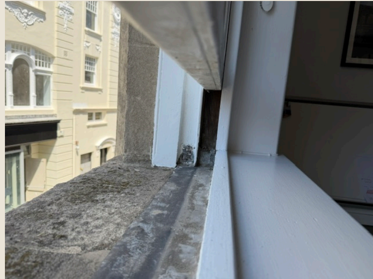
Figure 1 - Existing view of the cable, going through the window frame
