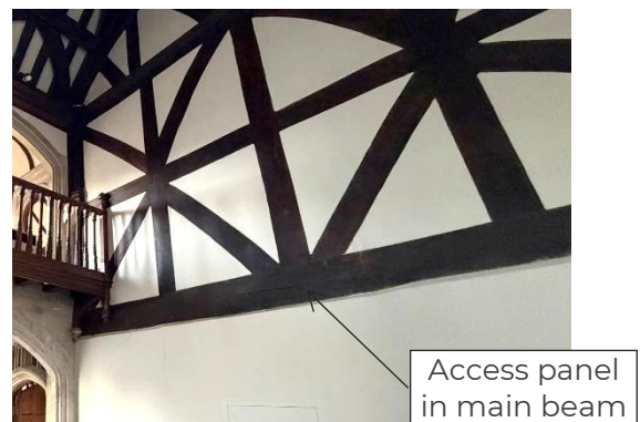
Figure 20 – timber access panel on opposite side to saddle
