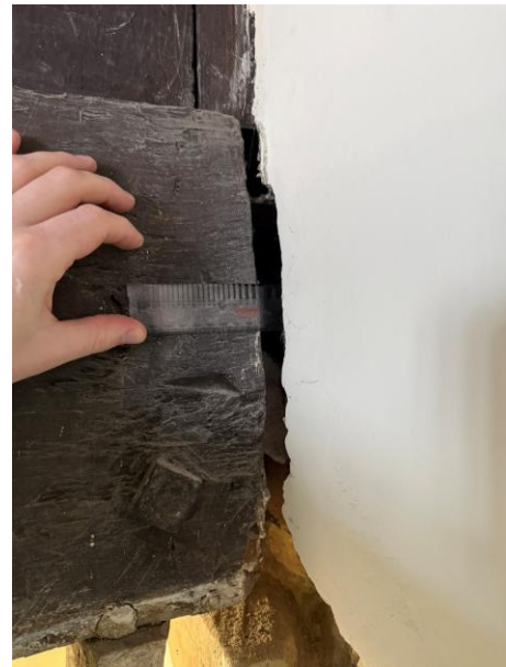
Figure 26 – deep void at north end of main beam viewed from Hall
