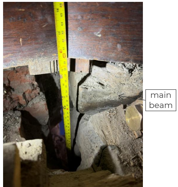
Figure 24 – void at end of main beam viewed from Solar
