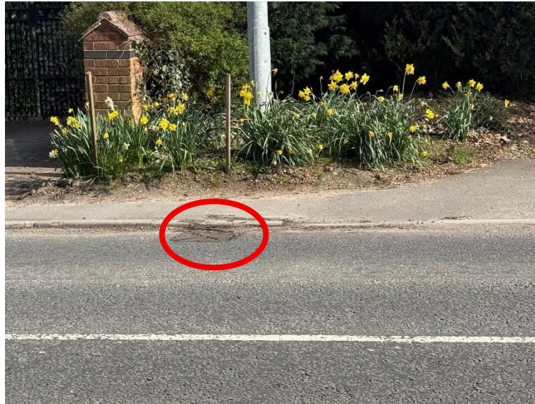
Image 4.2 – Existing gully in carriageway
