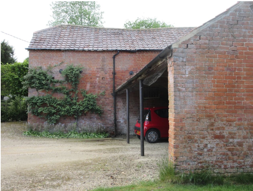
North elevation with high ridge deflection- note garage relies on main barn for stability
