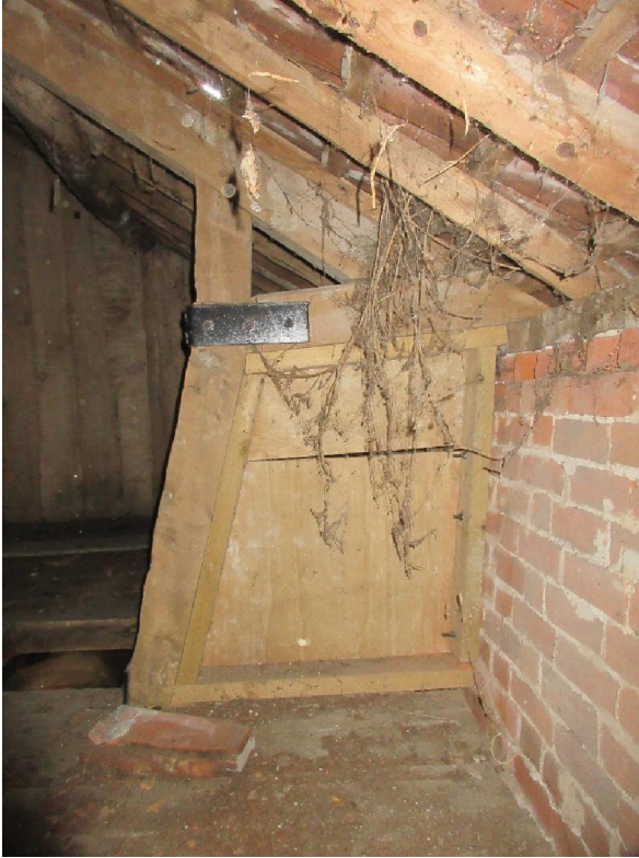
Eaves detail showing high lateral deflection and bent post (some are cracked)
