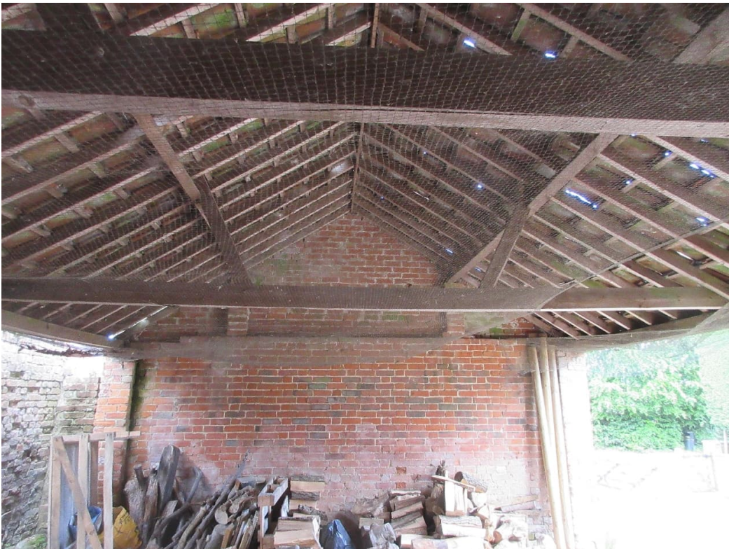
Internal garage roof tied rafters- note sag in tie beam due to inefficient connections
