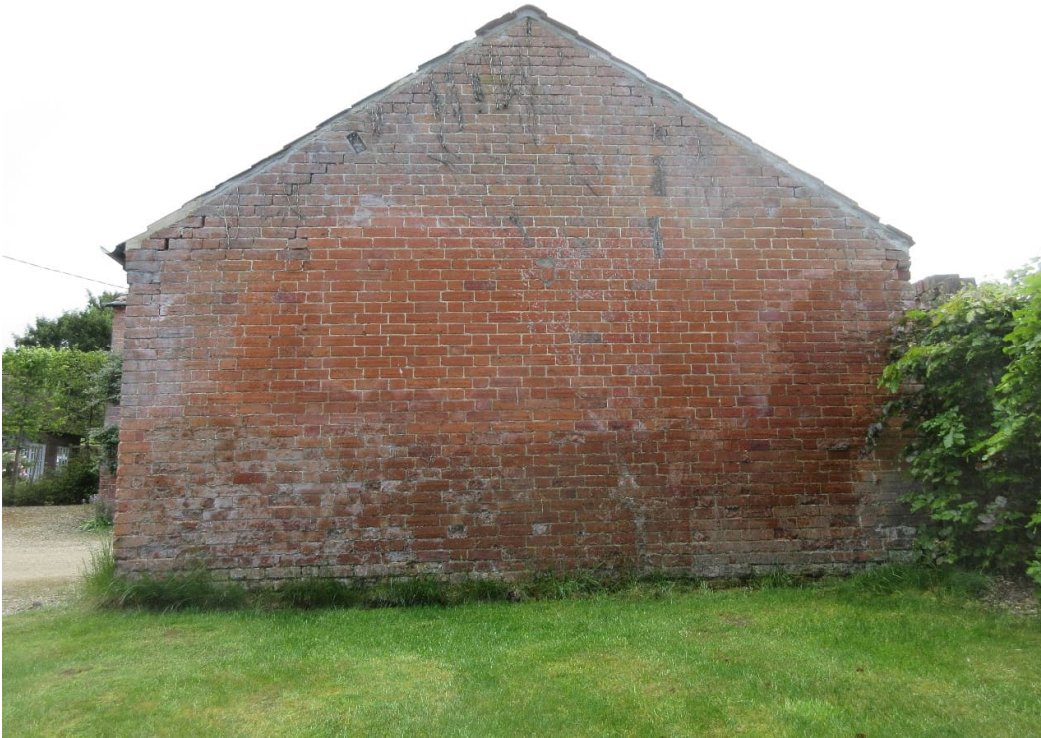
Garage end gable- high left hand side deflection and damage due to main barn movement
