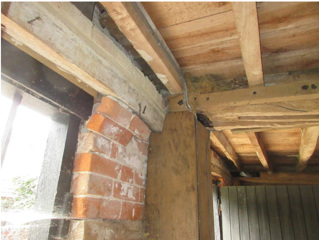
Failed beam bearing having pulled over the binder and 3 courses of bricks
