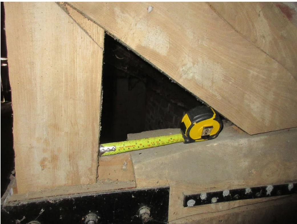
Detail showing 6cm tenon failure
