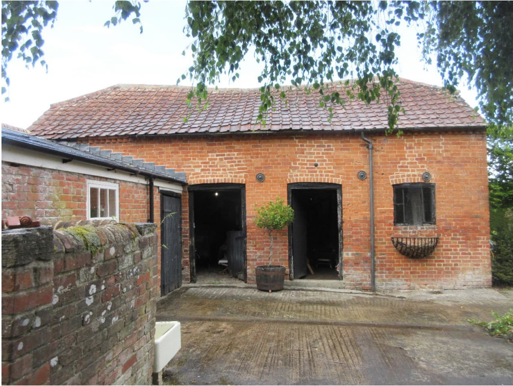
South Elevation Barn- note 3 brick arches and movement/ repairs
