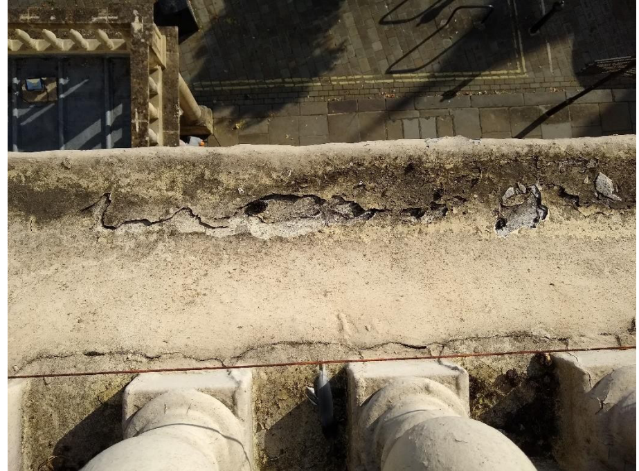
Figure 5: East elevation top of external wall showing paint spalling.
