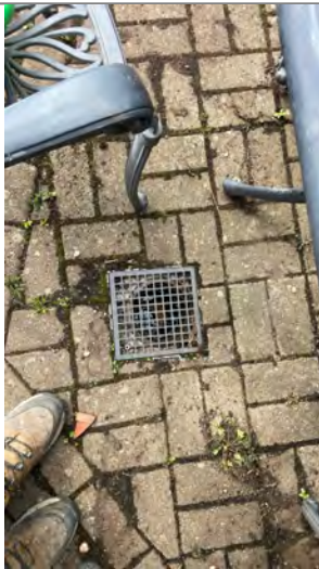
Other Site Photos: Gully 2
