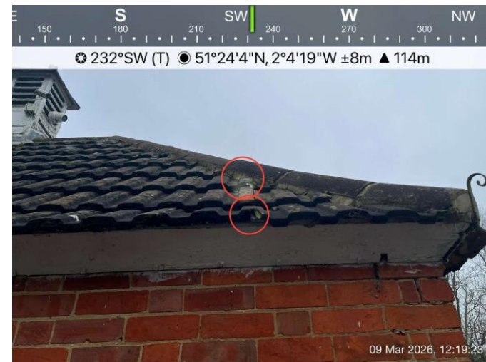
Lifted tiles on north elevation of B1
