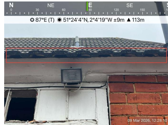
Gaps under edge tiles on west elevation of B1
