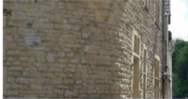
Exposed rubble on façade
