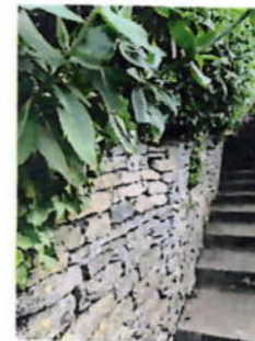
PLATE 3 - Bulge Lower Retaining Wall
