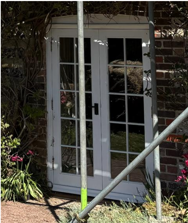
Front façade French doors – double-glazed replacements with applied glazing bars
