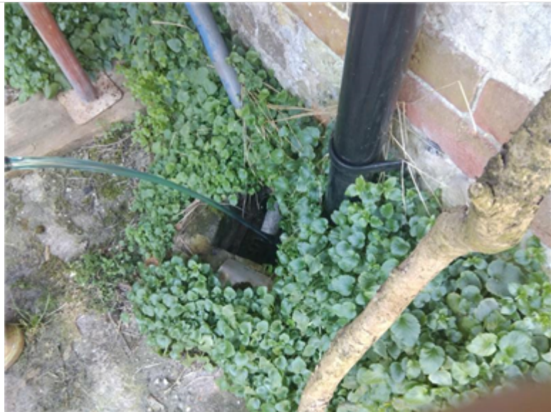
Photograph of dye test undertaken
