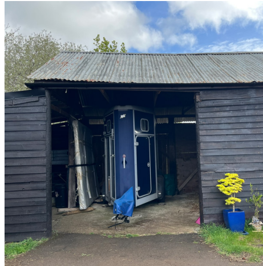
Outbuilding in need of re-roofing
