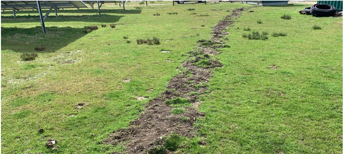
Trench During Wet Period
