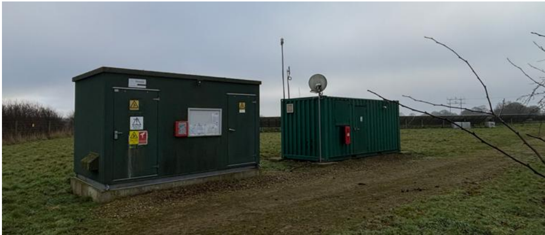
Photo 7: A Typical Item of Fixed Equipment
