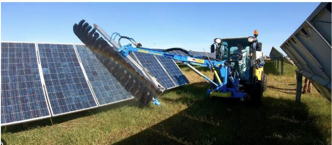
Cleaning of Solar Arrays
