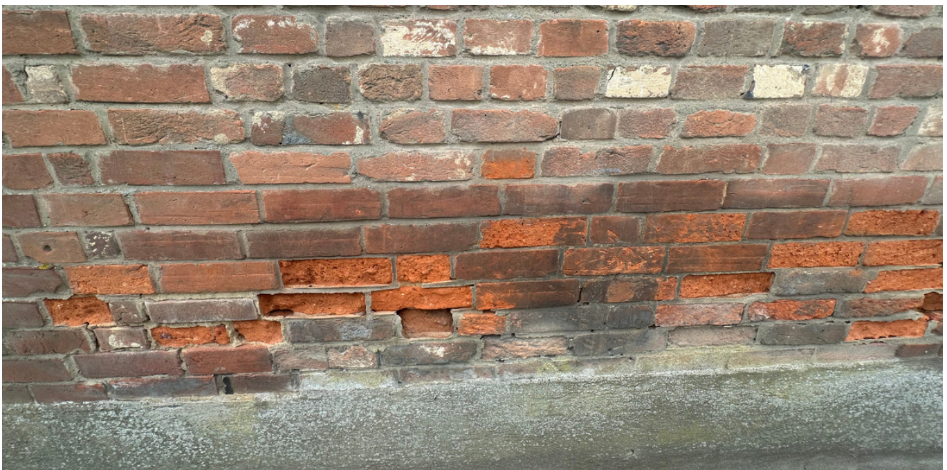
EXISTING NORTH WEST ELEVATION DAMAGED BRICKS
