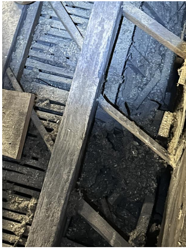
024 Area behind cornice detailing evidence of debris from timber shavings.
