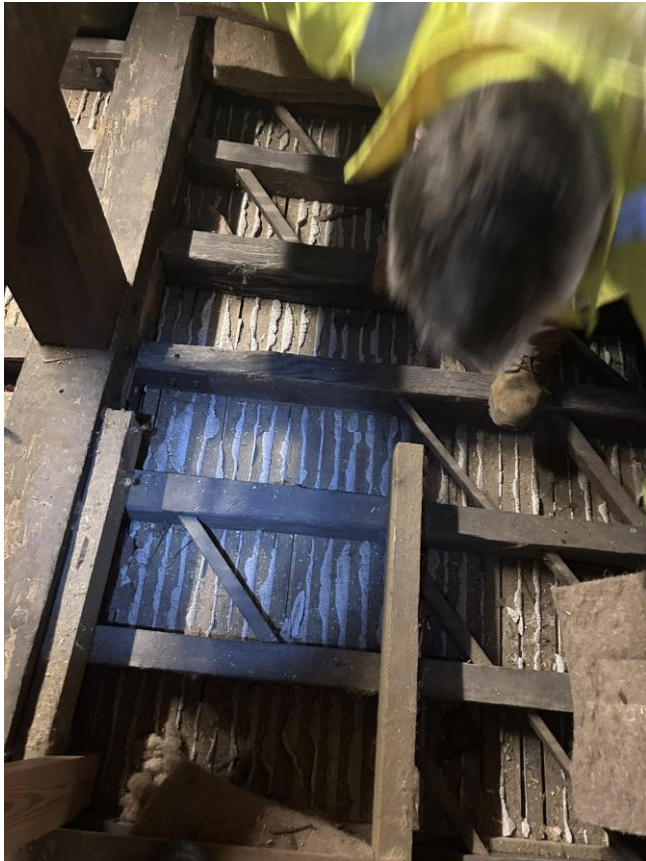
021 Area of medium risk appears to have some missing areas of key; however plaster still seems quite secure in arched part of ceiling void.
