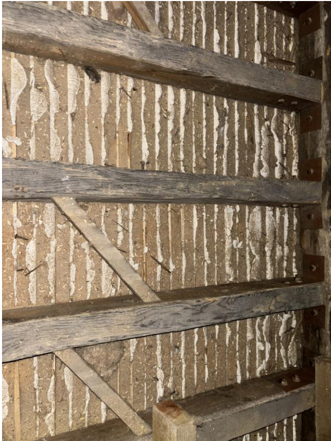
009 Medium risk zone, with no ply backing, some areas have a slight loss of key but this is in small, localised areas, with the plaster being still secure.
