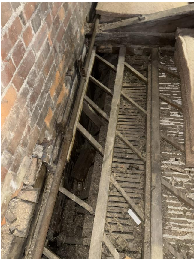
015 Another area behind corner area has some debris inside however not substantial.
