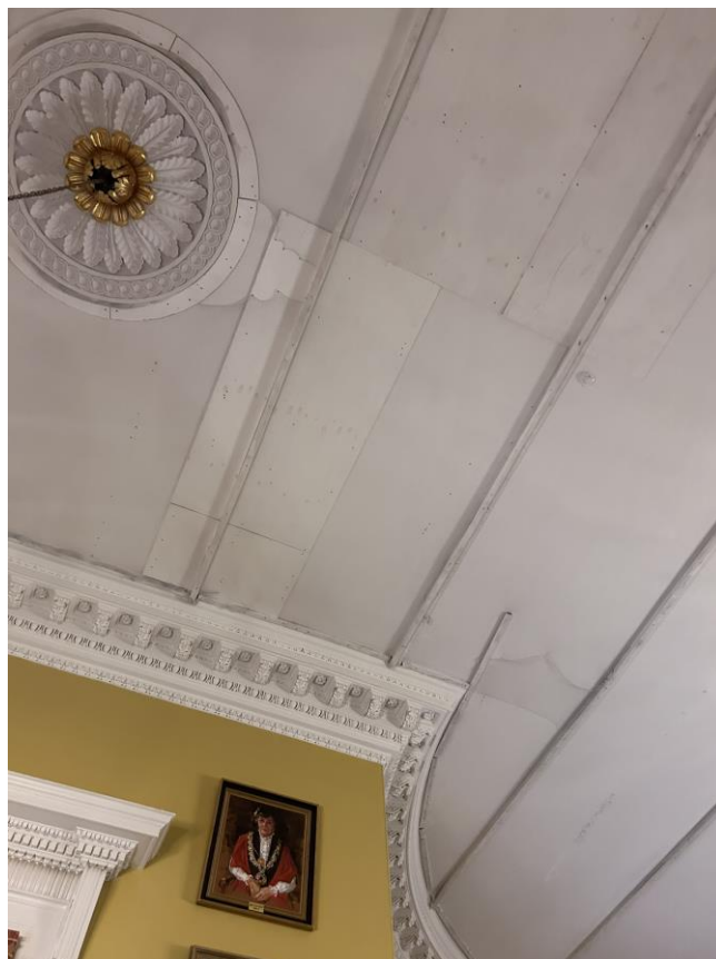
04 Area which has been previously repaired using ply boarding and netting with fixings from below appears to be well secure.
