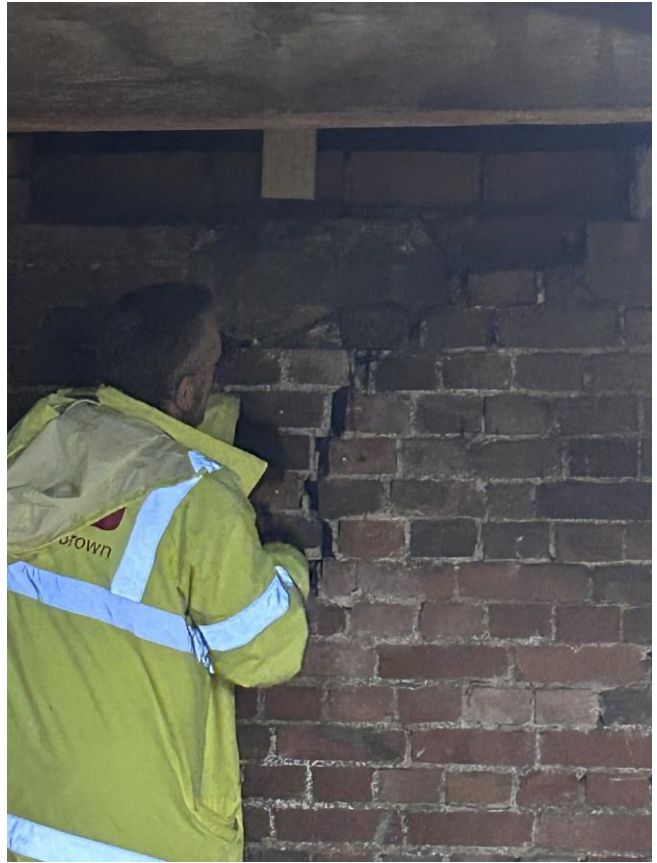
026 Taking measurements of existing tell-tales/crack monitoring on established fracture in brickwork.
