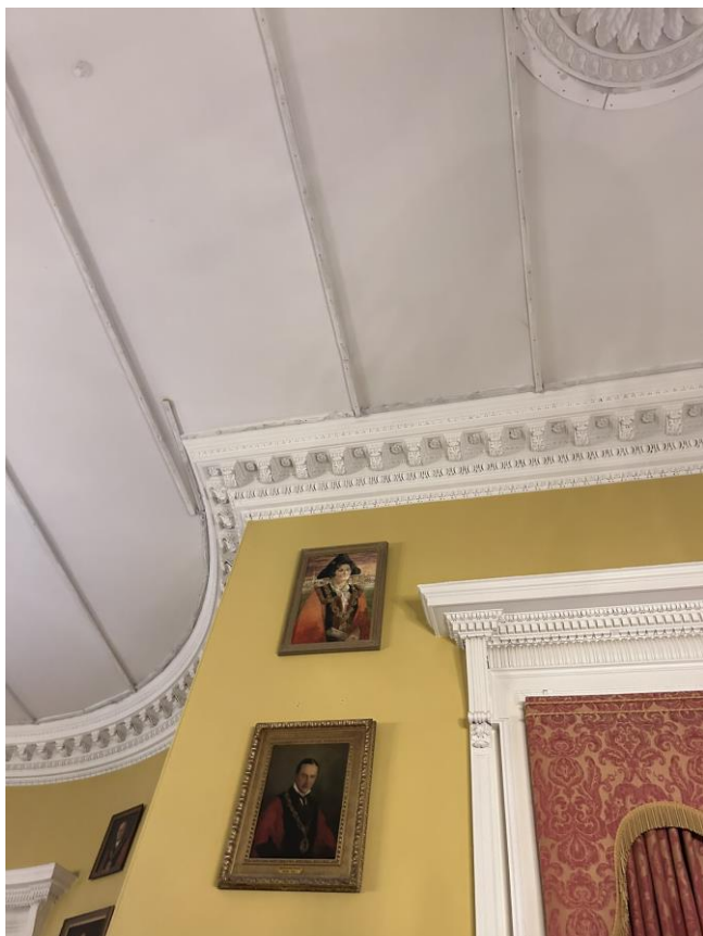
03 Area identified beneath crack in roof, no signs of cracking in the room below.
