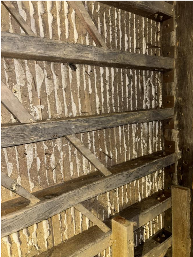
05 High risk zone identified, where key is more degraded than other areas, with ply backing been installed.
