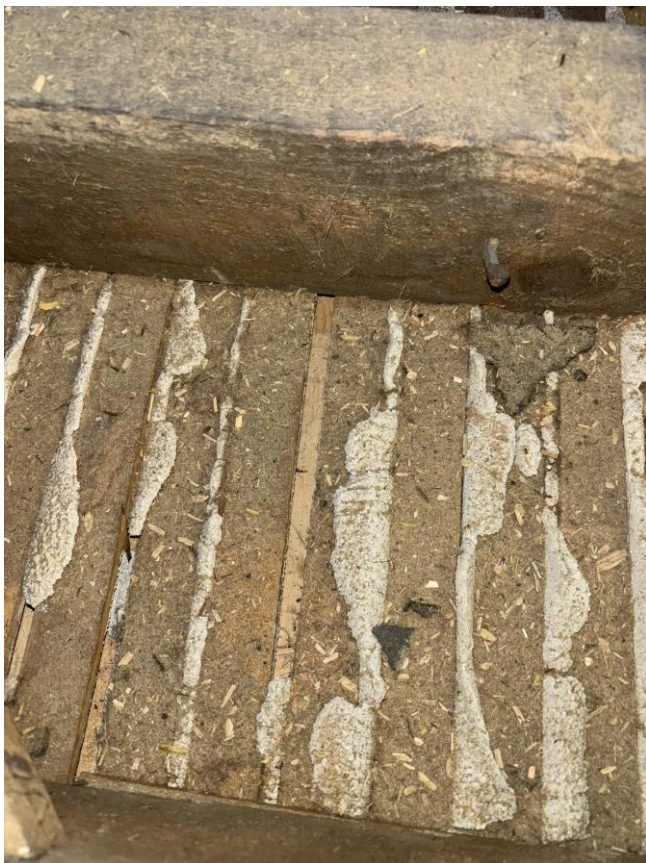
07 Area in high risk zone with loss of key (doesn't seem to have worsened).
