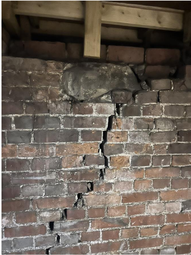
025 Large vertical crack on East elevation about 1.8m in length and the widest part being approx 35mm.
