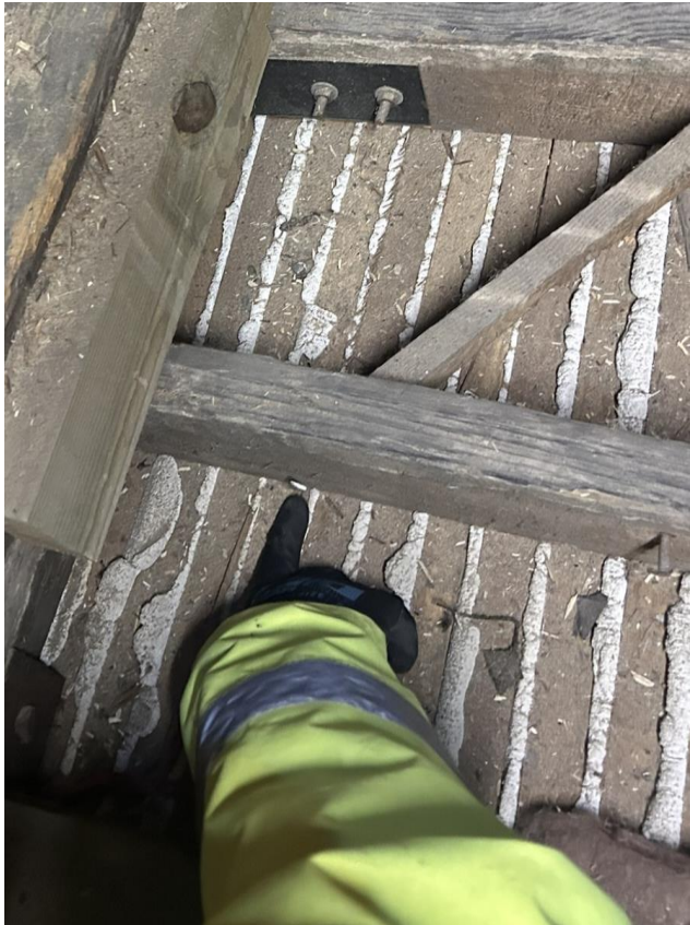
018 Approx 100mm fixings securing battens to underside of ceiling which in this case has missed joist.
