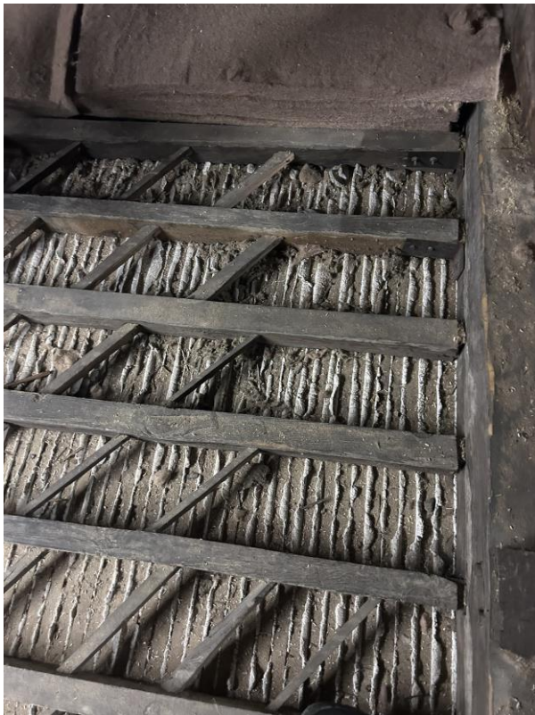
023 Low risk area key is well covered, the joists in some areas could do with some extra fixings as seemed to flex slightly while walking across them.
