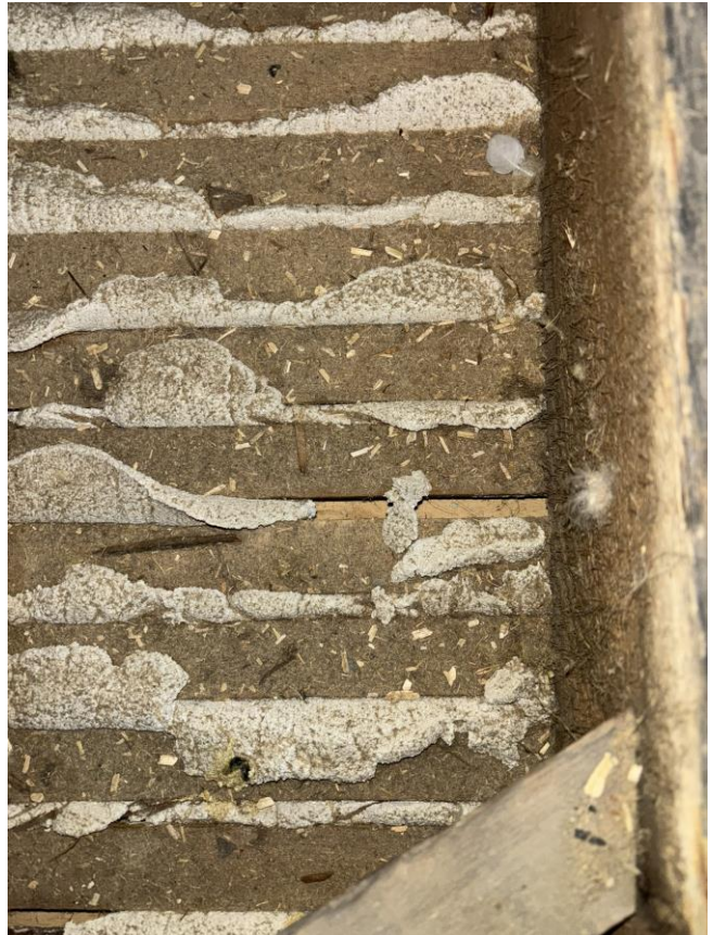
06 Evidence of ply backing has slight flex in areas however seems quite secure.
