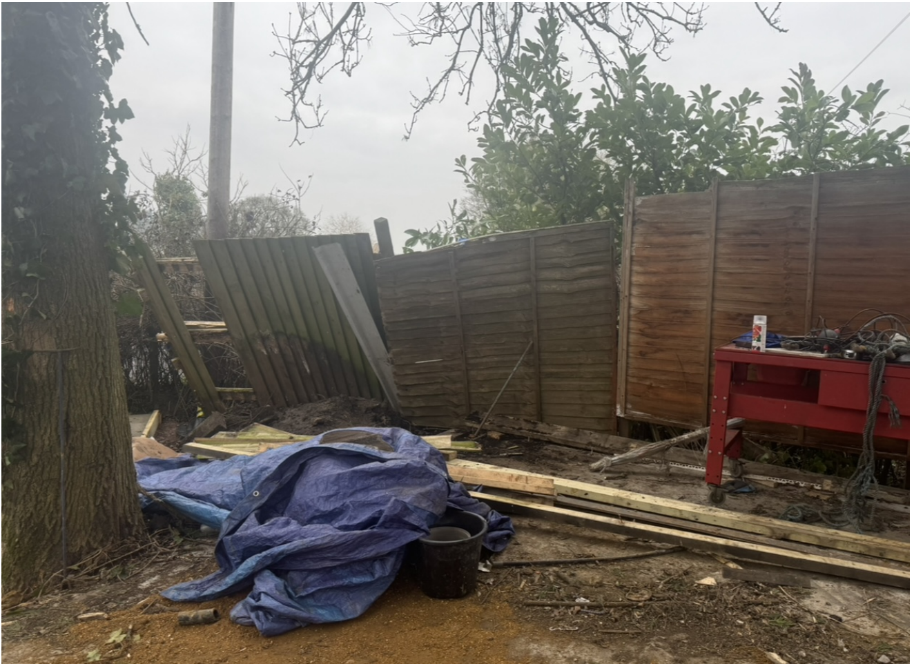
Former fence collapse - wider view of the previous boundary after collapse.
