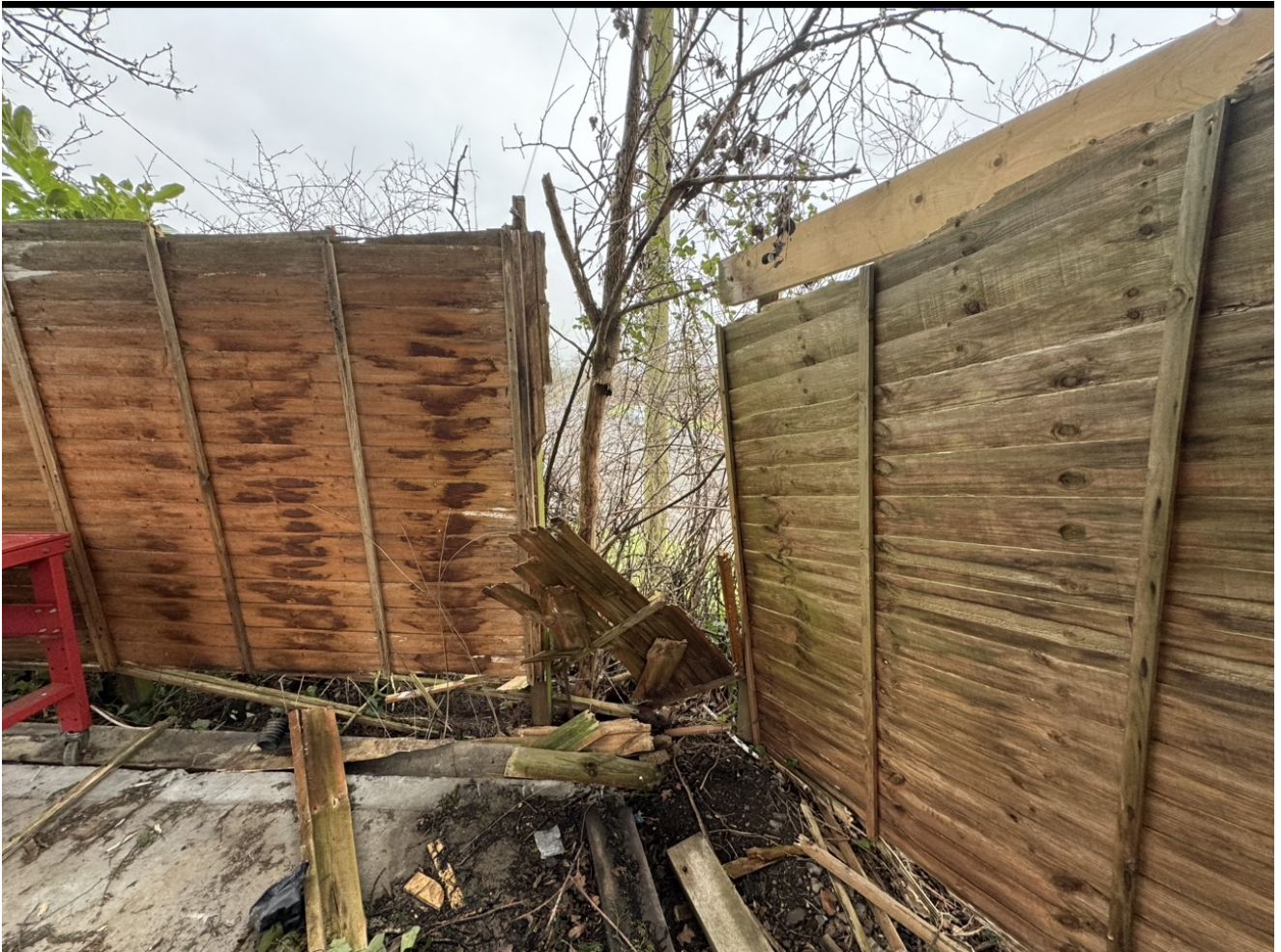
Former fence collapse - photograph showing the previous boundary in a failed and dangerous condition.
