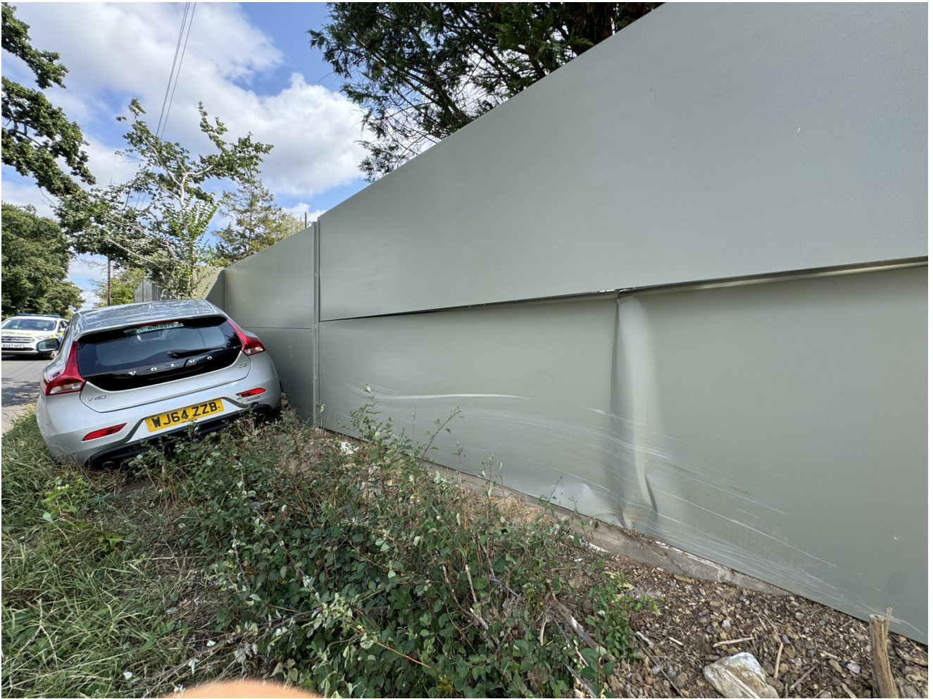
Photograph showing the vehicle lodged against the fence after the collision, demonstrating the impact on the boundary structure.
