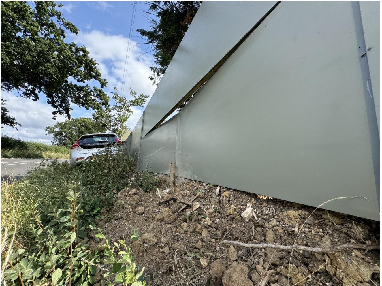
Low-angle photograph showing scrape and impact damage to the fence following the collision.
