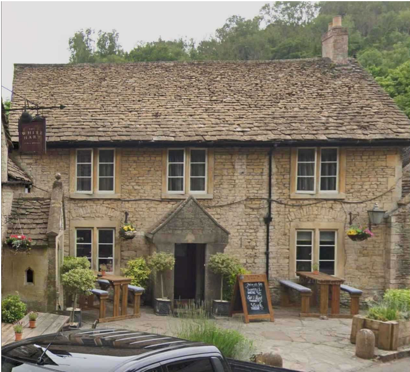
Pic.3 An image of the elevation shown in Pic.1 prior to the damage event (Google Images 2025). The porch structure outlined.
