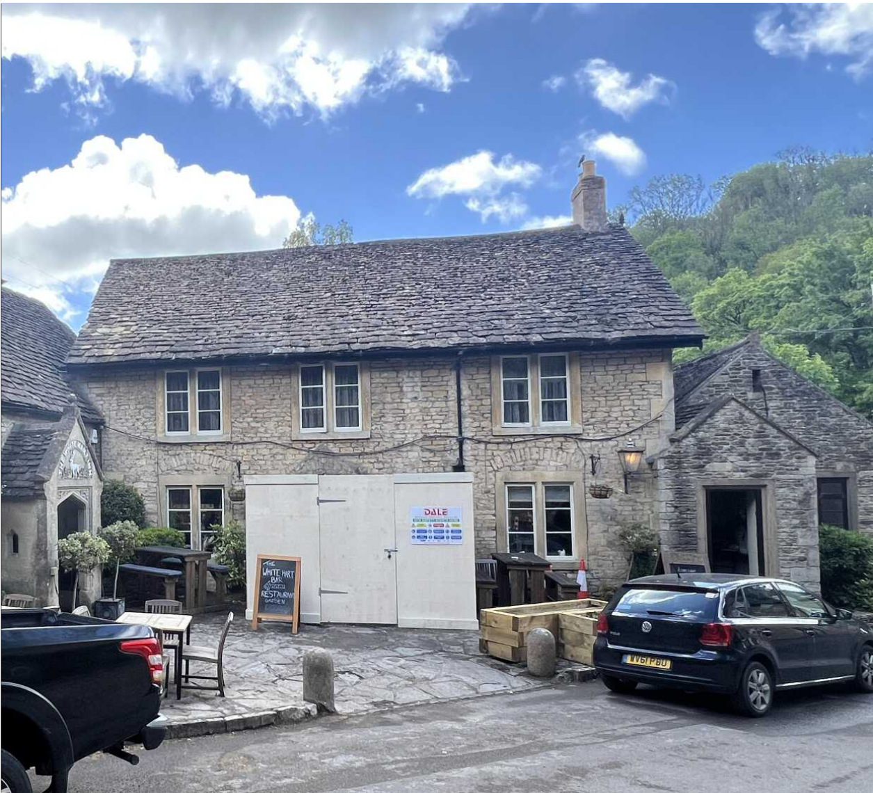
Pic:1 Highway facing elevation of The White Hart. The photograph was taken at the time on inspection on 13th May 2026. The plywood hoarding is enclosing the area of impact damage caused by vehicle collision.
