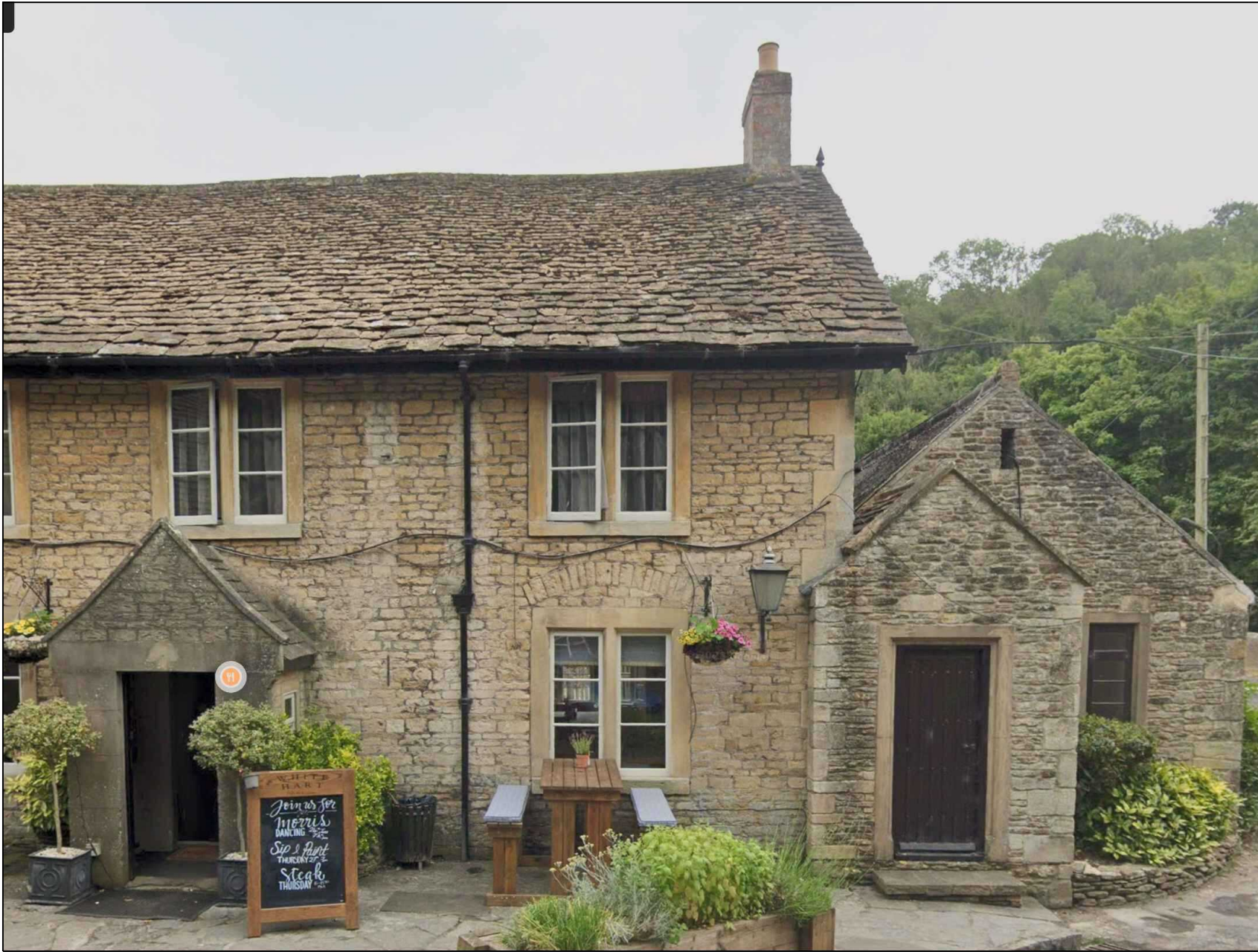
Pic.17 This elevation of the building had two projections, the one to the left side now removed following extensive damage. It has been suggested that the composition of the damaged porch was inferior to the surrounding elements, in that the stone effect was a render, the blocks were concrete and suchlike. The preference for rebuilding was that natural 'real' stone be considered in the design.
