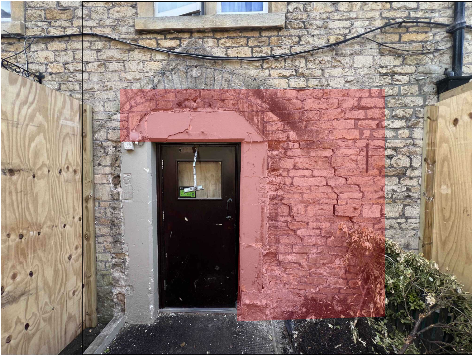
Pic:2 Internal view of the affected area inside the protective hoarding enclosure. The outline of the porch structure that was severely damaged by the impact is visible on the face of the main wall. The debris of the structure following collapse has been removed. The 'footprint' of the structure remains, as the walls below ground were left in place. The dimensions used as the basis for reconstruction have been taken from the remaining elements and the marks left on the building face. Highlighted area for rebuilding (details shown in separate document). Refer in conjunction Pic.5 - Pic.10.
