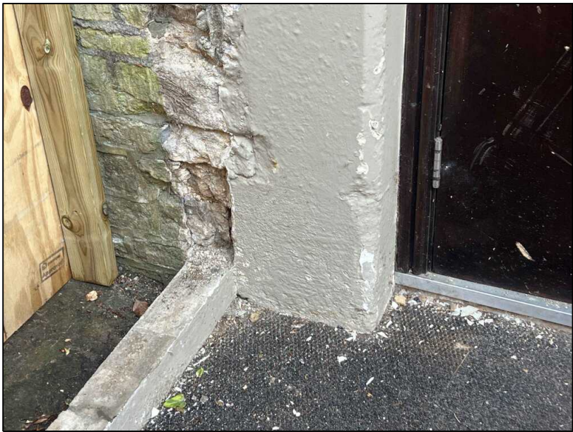
Pic.6 The wall to the left side of the opening is not exhibiting any significant damage. The position of the porch structure wall is clearly visible. There does not appear to be have been any mechanical tie between the porch structure wall and the main walls.
