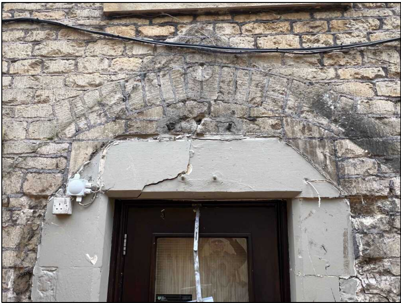
Pic.7 At the head of the opening there is a cut stone lintel beneath a stress relieving arch (or formerly there was a wider opening). The lintel has cracked and its structural capacity is no longer sufficient as a result.
