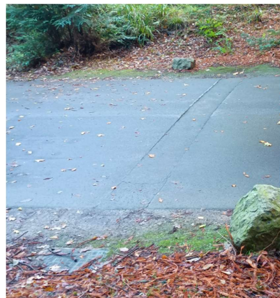
Figure 6: The location of the duct below the driveway adjacent T42.
