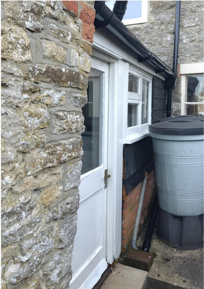
View of the existing, poor modern infill that presently houses the kitchen
