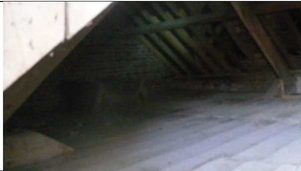
Intersection of roof frame with building 3 showing gaps between beams
