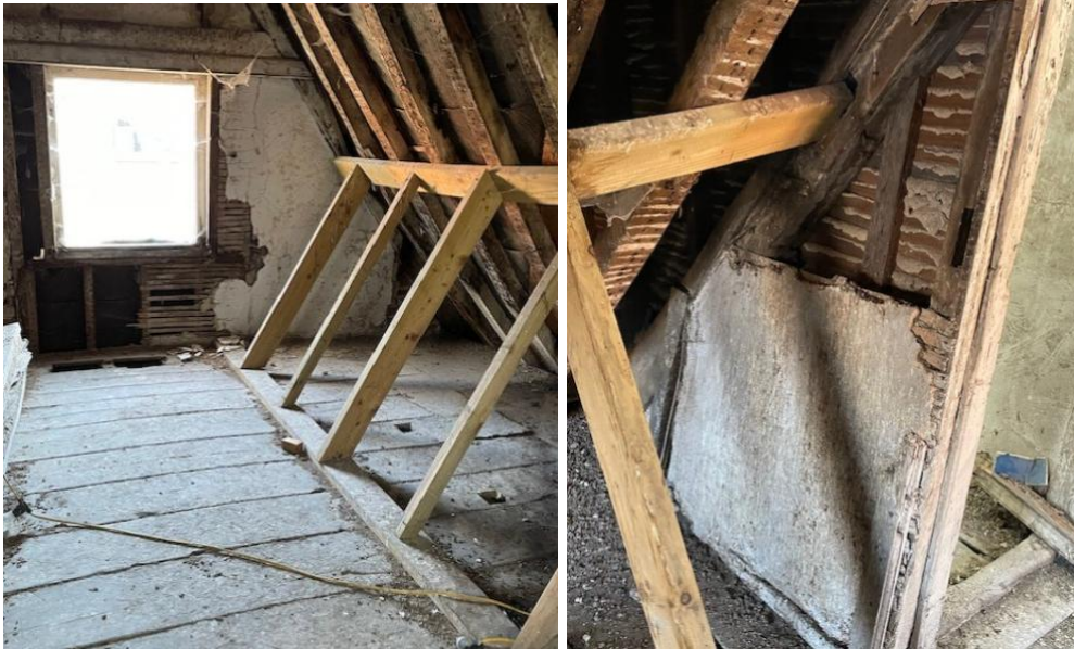
Photos in attic showing survival of L&P which should be repaired.
