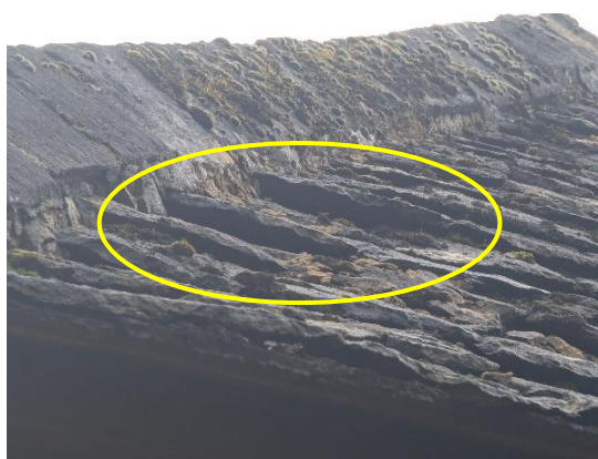
Figure 9. Potential access point beneath roof tiles of main dwelling
