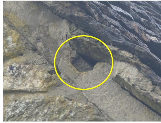
Figure 12. Crevice access point in the stonework
