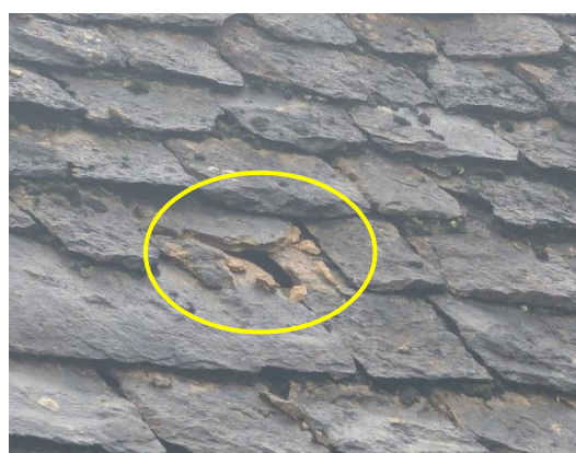
Figure 10. Broken roof tile providing potential access point
