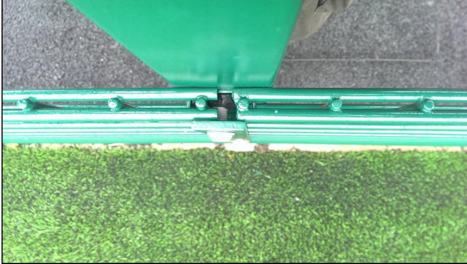
Figure 10: Image showing neoprene isolators
