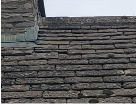
Photo 7: An example of the low number of gaps identified beneath the imitation stone tiles.
