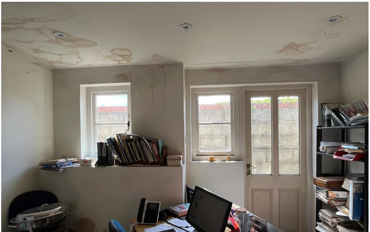
View of office below rear lean-to roof, showing staining as a result of leaks/water ingress caused by gaps in pantiles above and pitch of roof being about half that recommended for traditional pantiles. The proposals address this issue.
