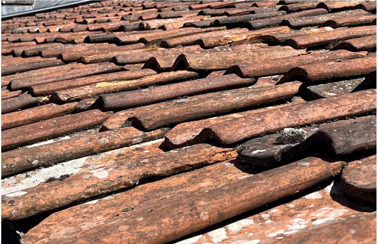
Detail of existing pantiles to rear lean-to roof, showing gaps between tiles and degradation of tiles which, together with the low pitch of the roof, are allowing rain ingress into the rooms below.
