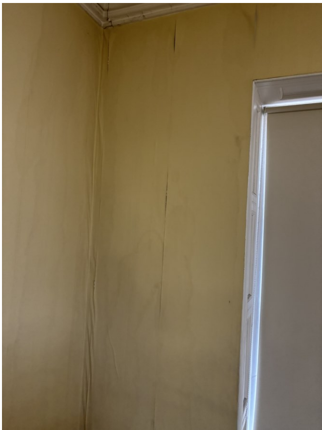
P37 – Signs of previous water ingress on South wall of Oak Court.
