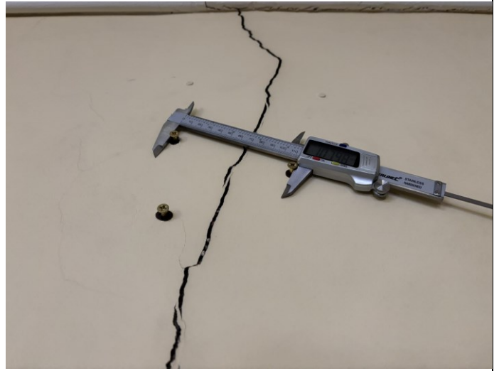
P32 – Digital callipers used to record crack width on North wall.
