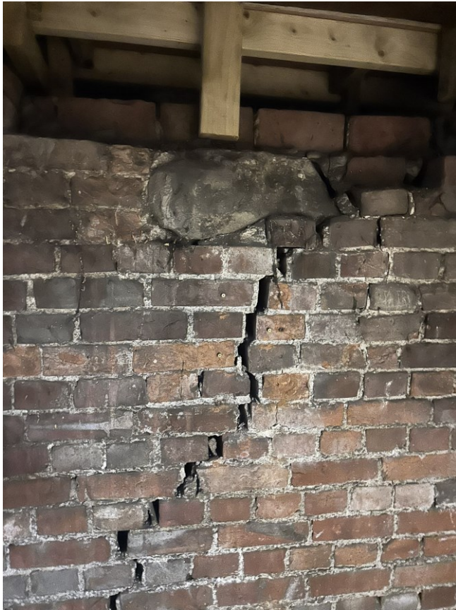
P55 – Crack through brickwork likely caused due to stress from roof.
