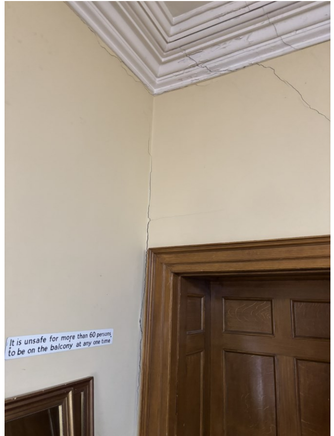
P24 – Evidence of door dropped due to structural crack.
