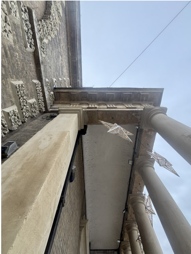
P1 - Crack can be seen Portico.
