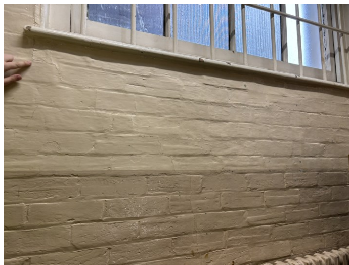
P52 – Crack through course and brickwork underneath Crittle windows.
