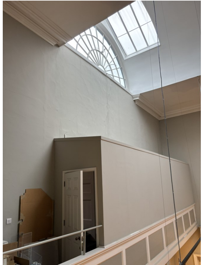
P20 – High level view of the Crown Court east wall showing vertical cracking extending down from the arched rooflight, consistent with the principal crack line observed through multiple levels of the building.
