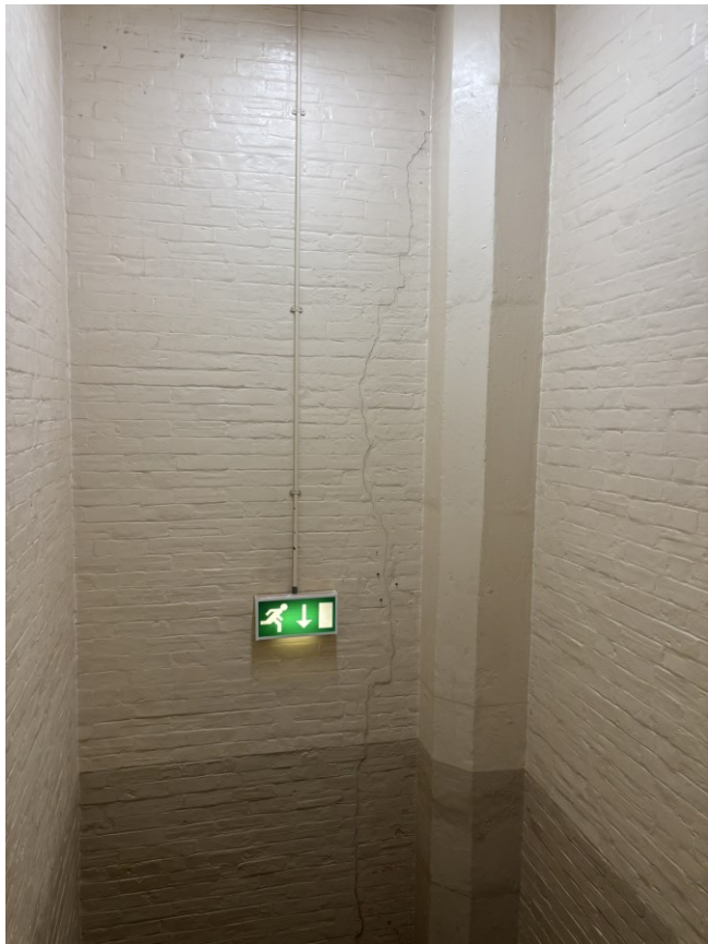
P43 – Overview of crack in staircase.
