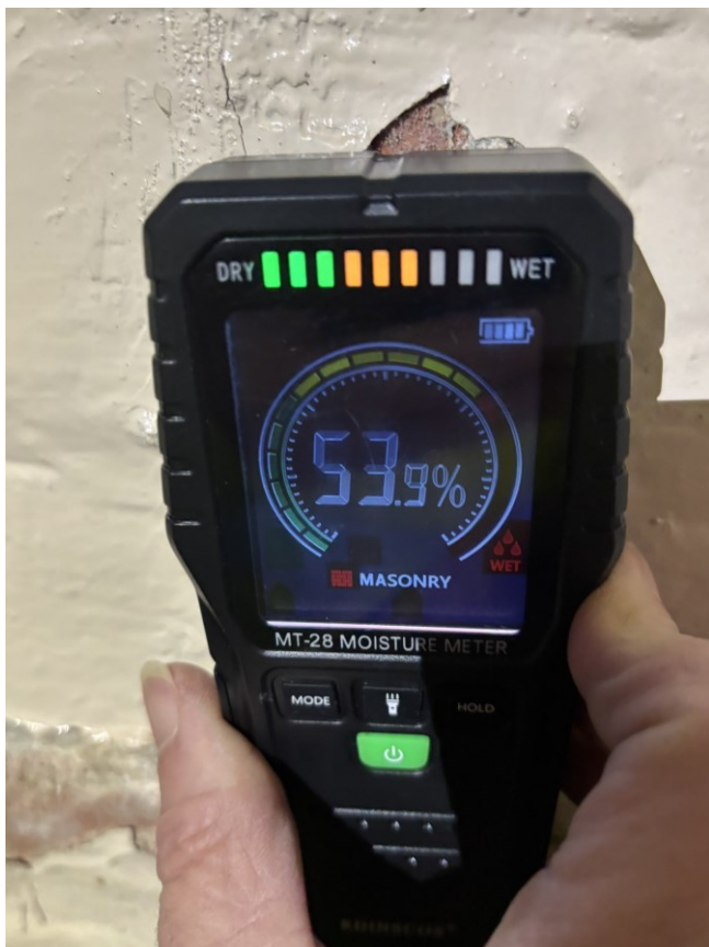
P49 – Elevated readings of moisture levels around flue.
