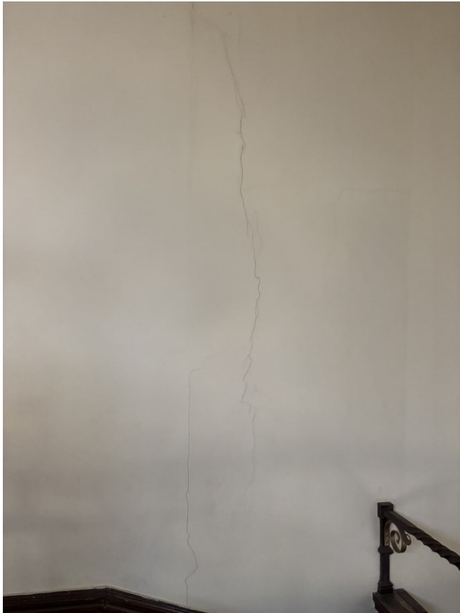
P35 – Hairline cracking observed on South wall.
