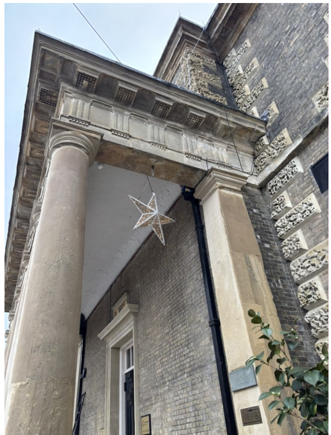
P8 - Crack on opposing entablature side filled in with a lime putty.
