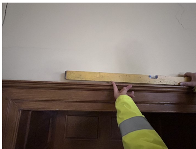
P30 – Door frame has dropped approx 30mm.
