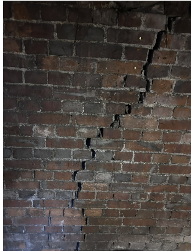
P56 – Crack through brickwork likely caused due to stress from roof.
