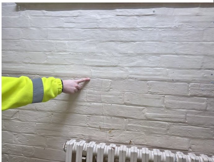
P51 – Crack through course and brickwork underneath Crittle windows.
