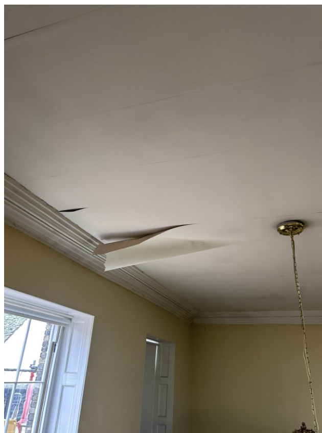
P42 – Paper sheets on ceiling loose.
