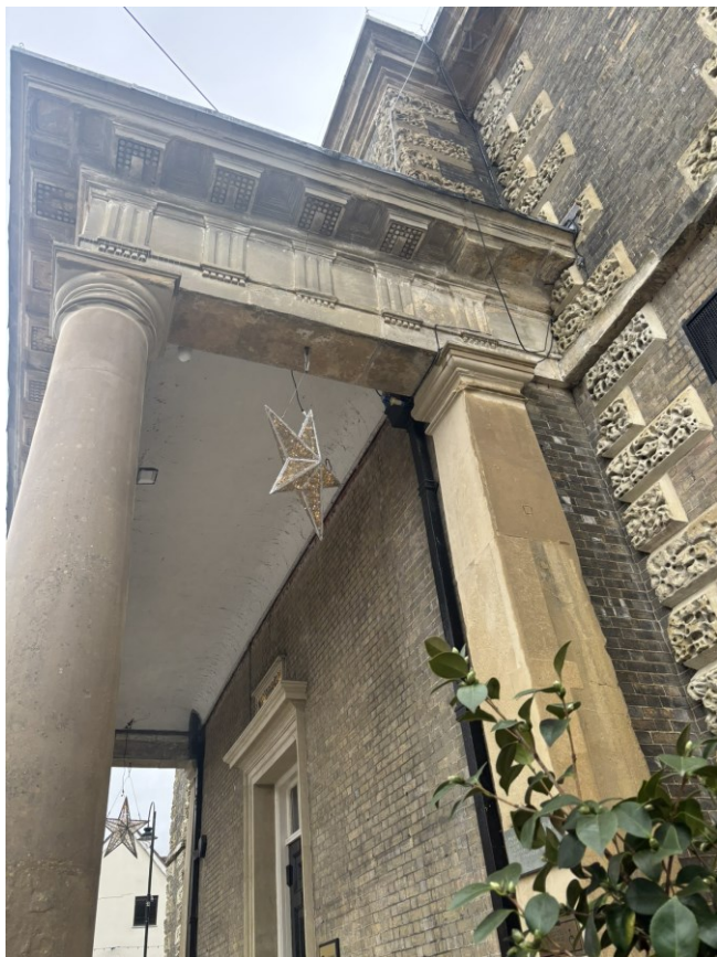
P7 – Crack on opposing side filled in with a putty.
