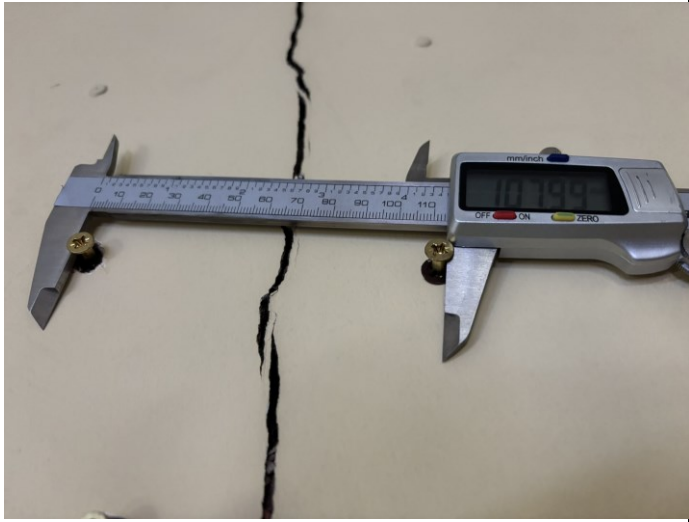
P31 – Digital callipers used to record crack width on North wall.
