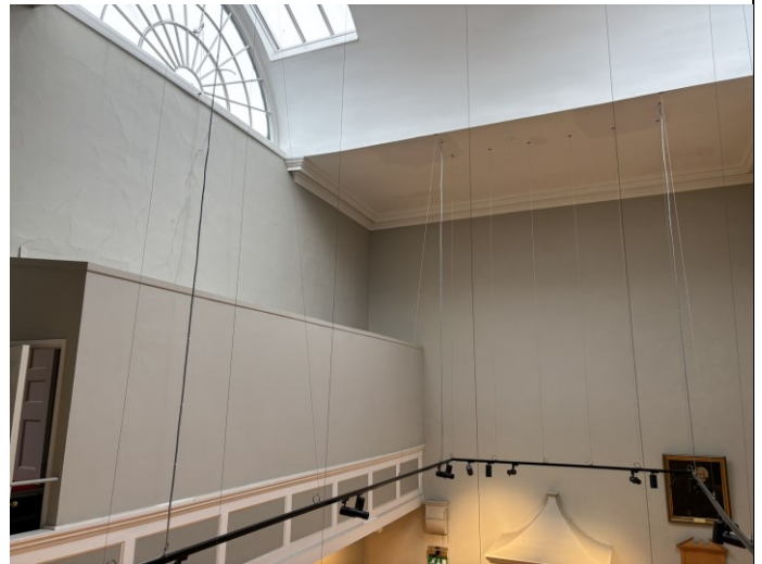
P22 – Principle cracks are restricted to underneath the arched window and extend below.
