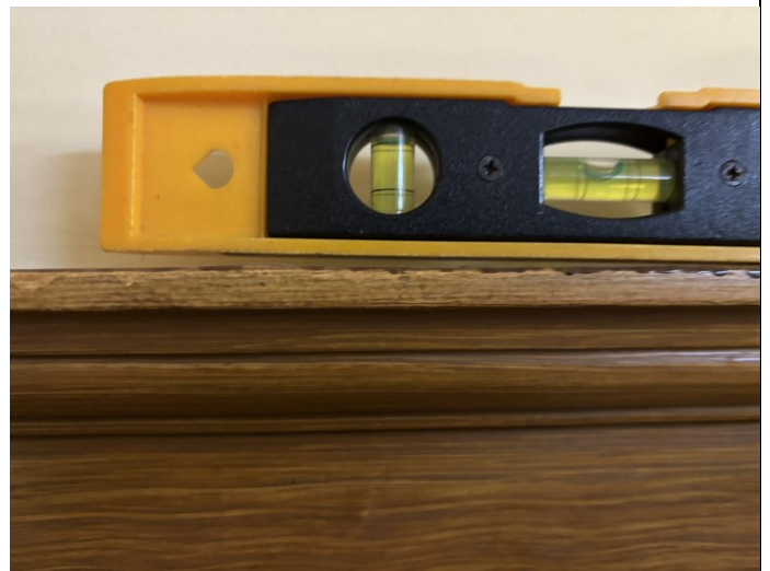
P26 – Evidence of door dropped.
