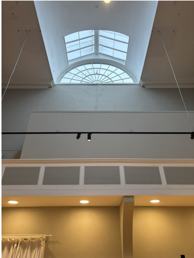
P19 – Structural Crack as seen on East wall.
