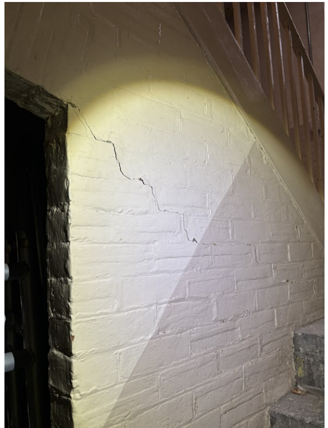
P48 – Stepped crack through course under staircase.
