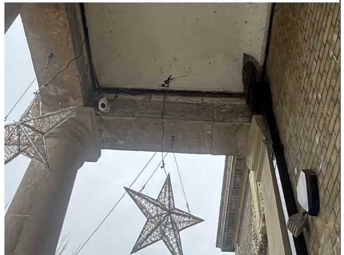
P4 - Overview of crack from under Portico.
