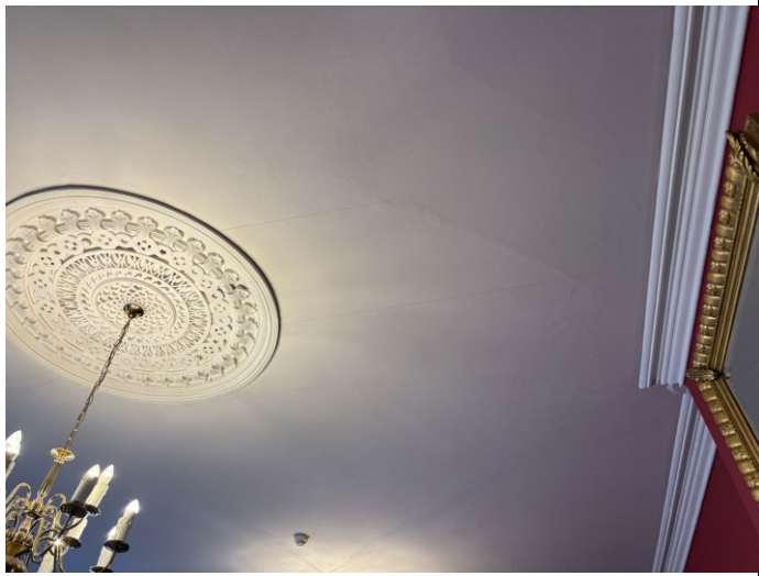
P11 – Hairline crack extends through rose to the other side of the room in a horizontal line.
