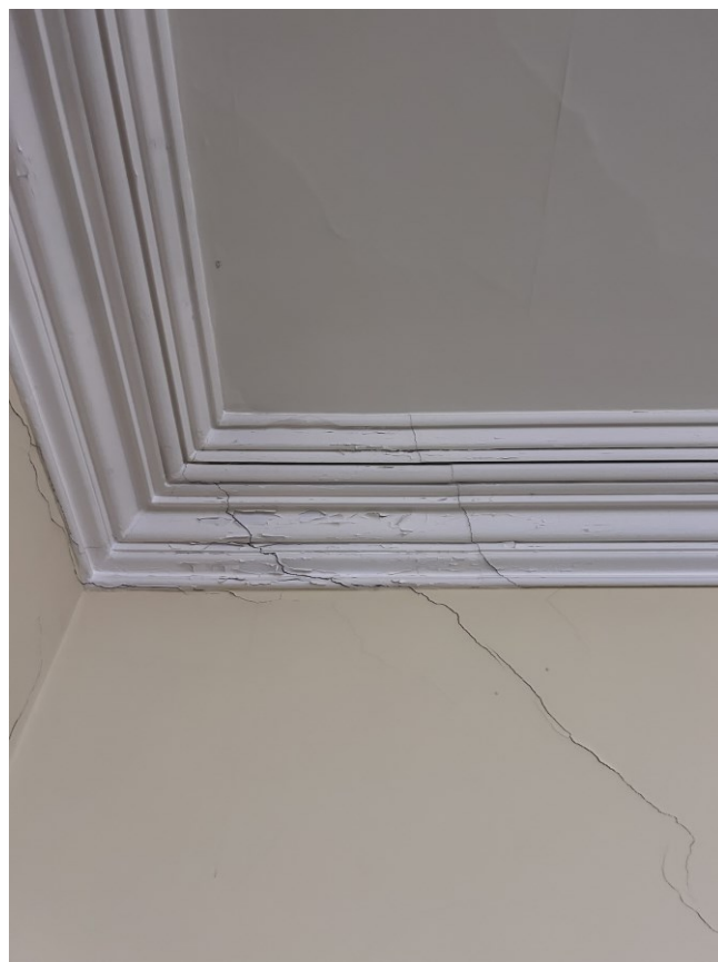
P28 – Hairline cracking coming off of principle crack.
