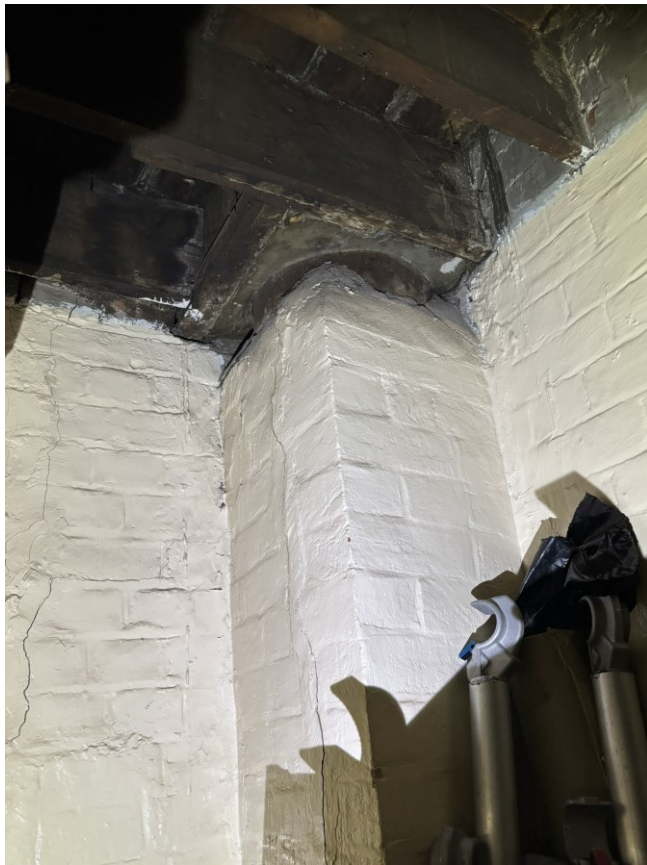
P47 – Evidence of corrosion on flue.
