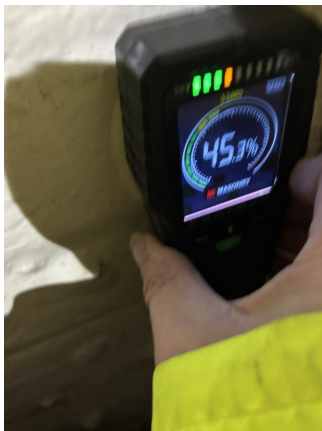
P54 – Elevated readings of moisture levels around flue.
