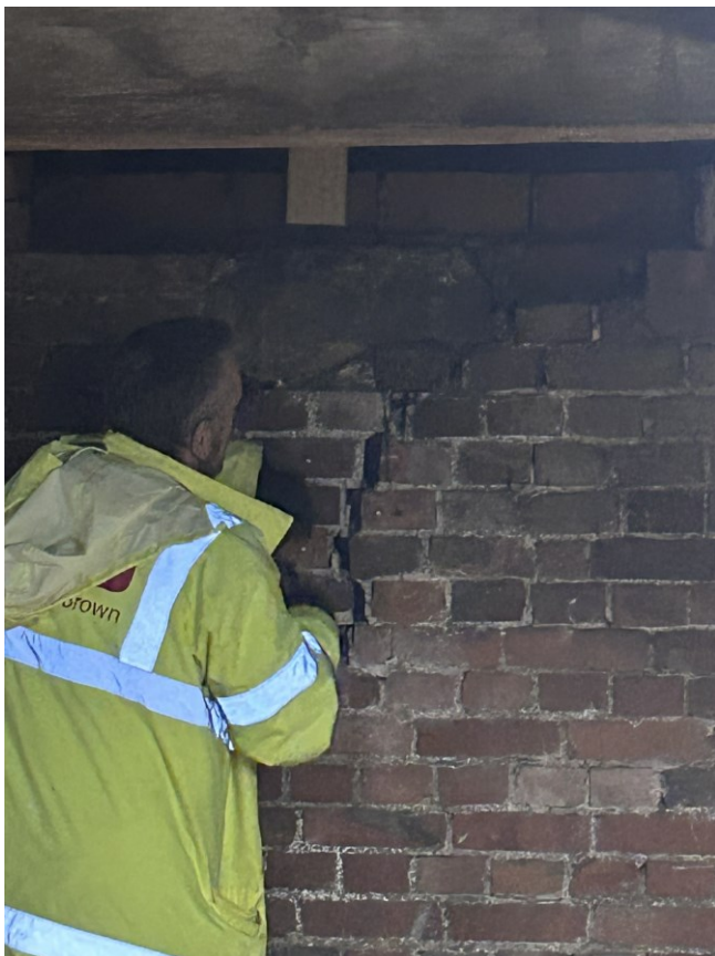
P57 – Crack width is 35mm at widest point.
