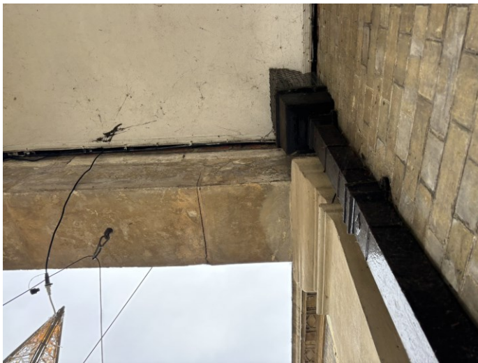
P3 - Close up of compressive crack in Portico.
