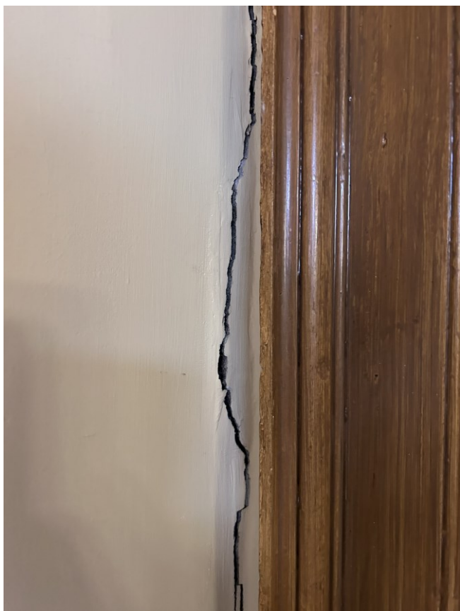
P27 – Close up of structural crack behind door frame.
