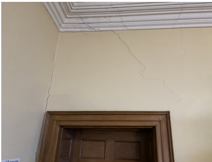
P25 – Overview of principle crack visible.
