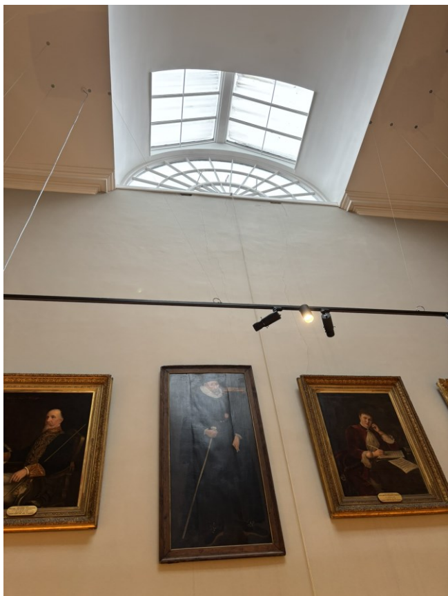
P17 – Longest crack here extends approx 7.7M
