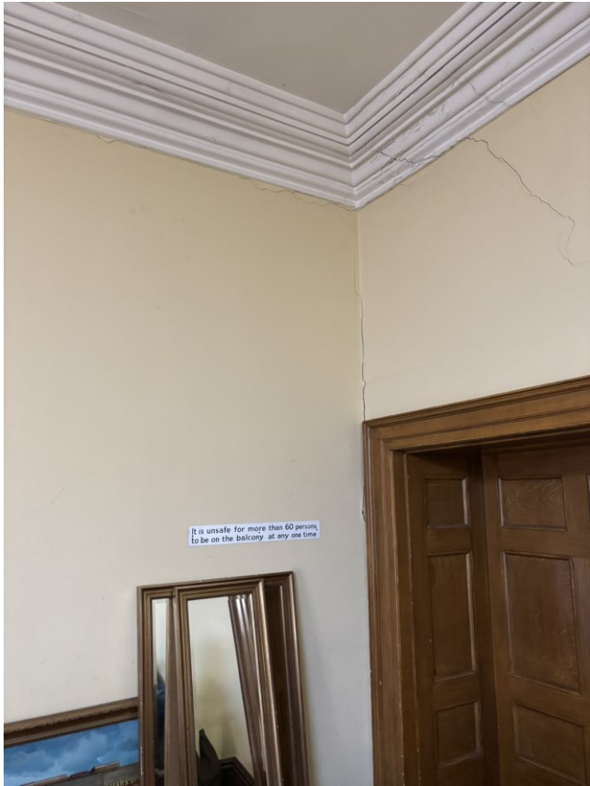
P23 – Principle crack observed in NW corner of room.
