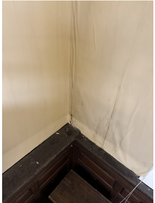
P36 – Signs of previous water ingress on South wall of Oak Court.
