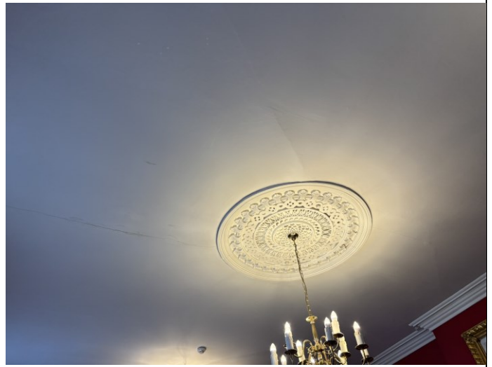
P10 – Hairline cracking in ceiling going to decorative rose.
