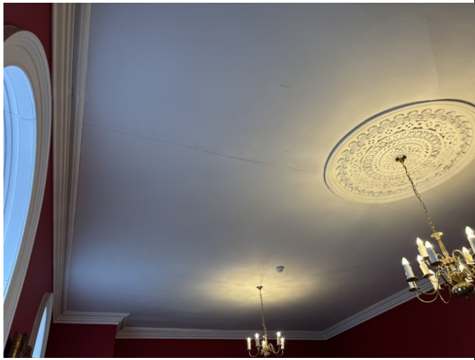
P9 – Hairline cracking in ceiling going to decorative rose.
