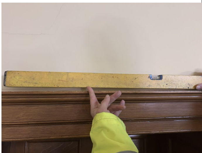
P29 – Door frame has dropped approx 30mm.
