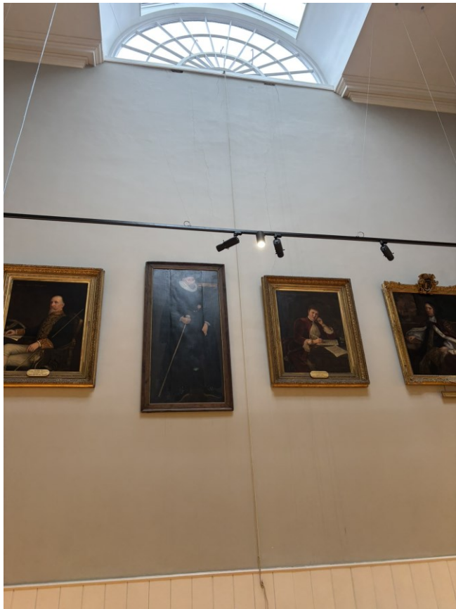
P15 – Various hairline cracks on West wall.
