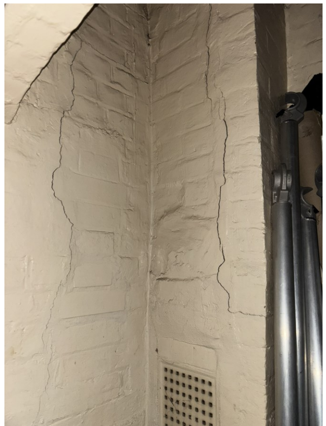
P46 – Cracking extending beneath staircase and further on flue.
