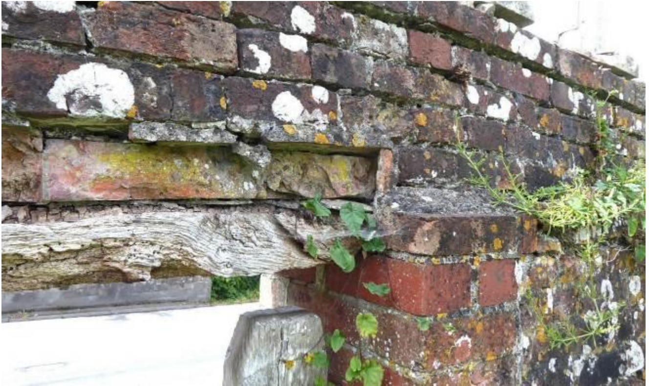
Upper wall thickness reduction (west side from field)
