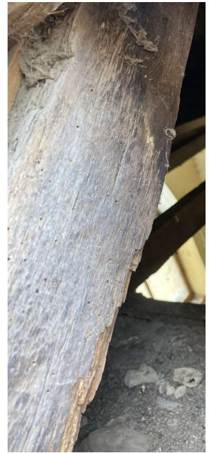
Roof timbers showing signs of woodboring insect attack. All existing timbers to be treated
