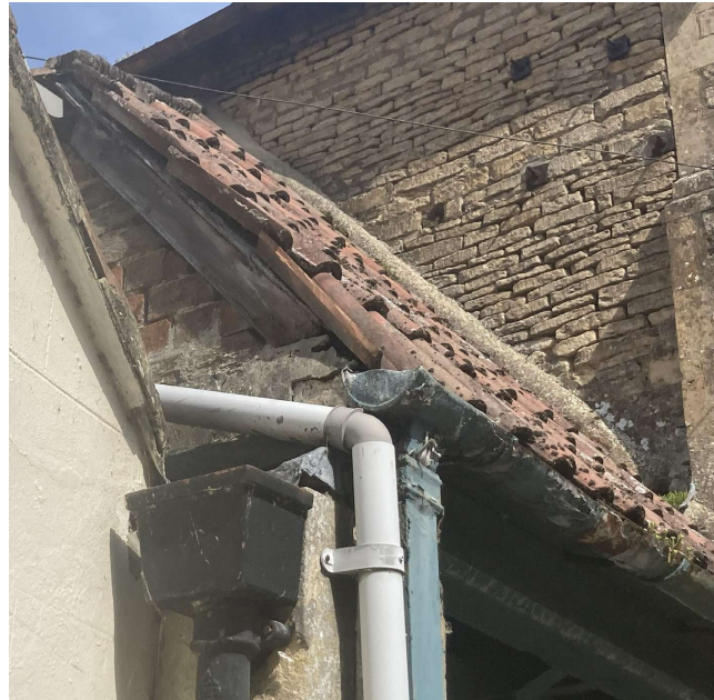
Existing timber to the verge of the ambulance station roof to be replaced. Mortar fillet also to be replaced with a lime mortar fillet
