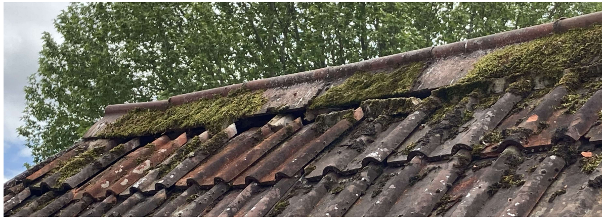
The existing roll top ridge is heavily covered in moss and the tiles are loose with the mortar bedding missing or loose. The existing roof is in poor condition with numerous slipped tiles especially to the north elevation, cracked and broken tiles are also evident across the roof across the roof slopes. There is also decay evident to some of the roof timbers although most look to be in adequate condition. These are to be inspected by a structural engineer
