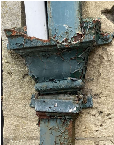
Existing gutters and downpipes to the east elevation of the ambulance station. The existing cast iron has degraded and broken off beyond repair and will need to be replaced along with the upvc for Heritage cast aluminium half round profile to the gutter and a square downpipe and hopper to match the existing as closely as possible.
