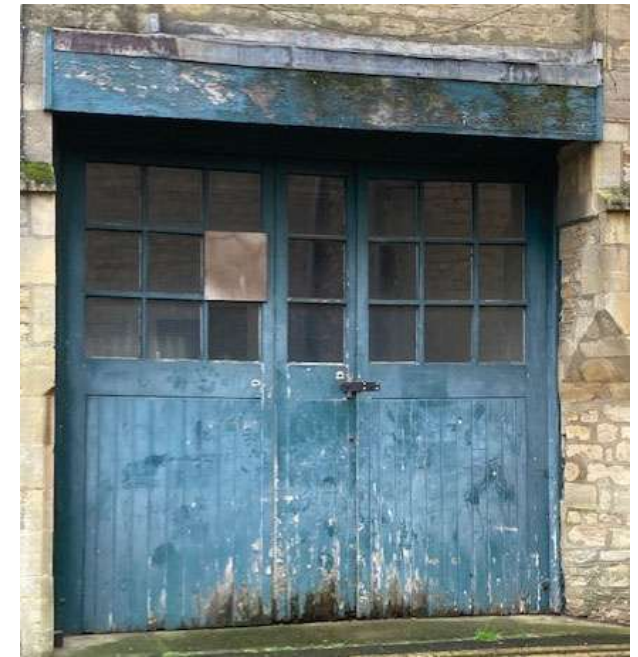
Existing main doors to the fire station. Doors to be sanded back. The timber to the bottom edge of the doors is rotten. This will need to be cut out and new timber scarfed in. Missing glazing to be replaced with new panes of single glazing to match the existing. Timber panel above the doors to be replaced with new. Lead flashing to be carefully removed and replaced with new. Prime and paint to match the existing. New hardware required.
