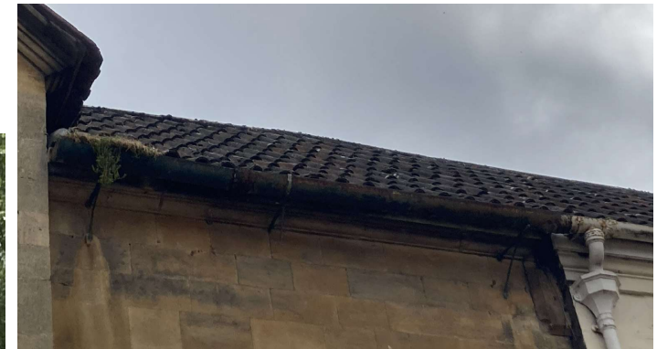
Existing cast iron gutter on rise and fall brackets has vegetation in and is in poor condition and needs to be replaced with new Heritage cast aluminium half round in profile.
