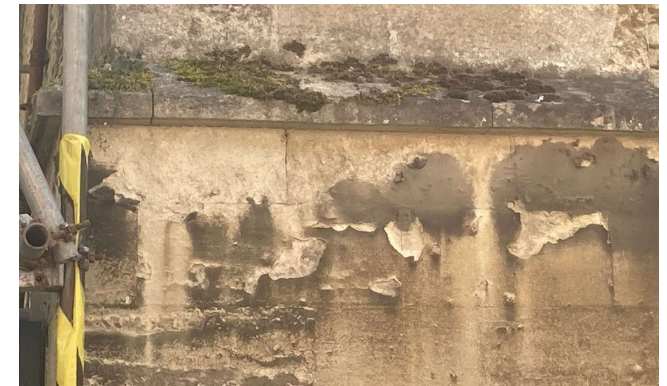
All moss to be carefully brushed off of the buildings surfaces where possible. Any vegetation to be removed.
