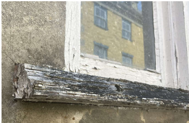
Existing small window needs a new timber sill. To be in hardwood, painted to match the existing
