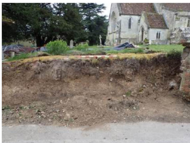
Figure 2. Location of collapsed wall (1m scale, looking S)
