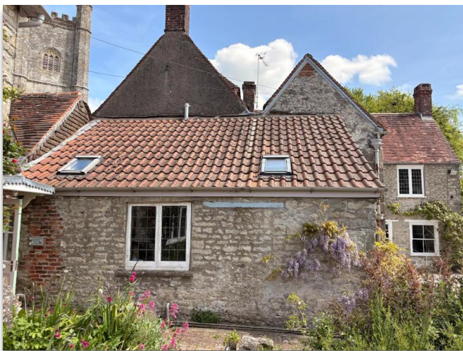
Figure 33. West elevation of existing kitchen; evidence of former opening (beneath lintel); anomalies in stone, evidence of straight joint.
