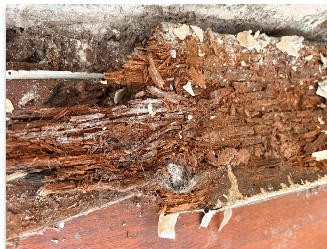
Figure 40. Section of drawing room skirting board, demonstrating level of decay.
