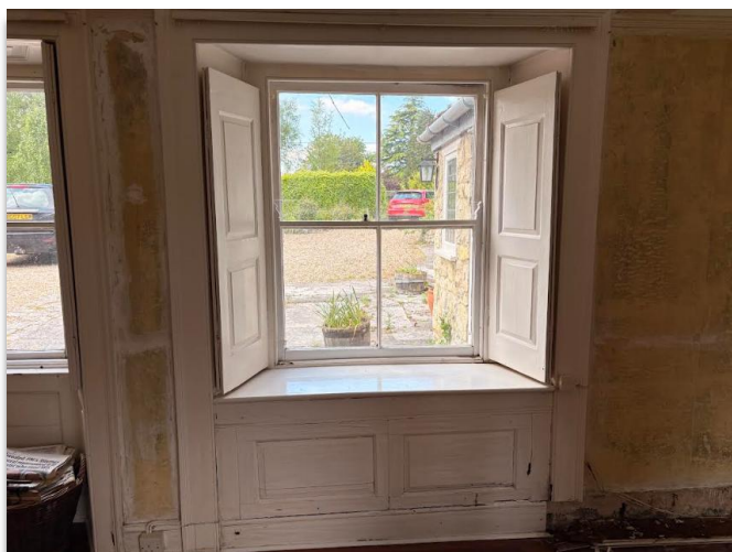
Figure 39. West window; panelling and skirting damp, suffering rot.
