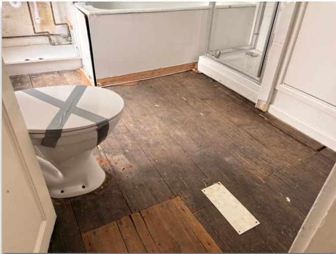
Figure 51. First floor bathroom. Ad hoc timber replacement.
