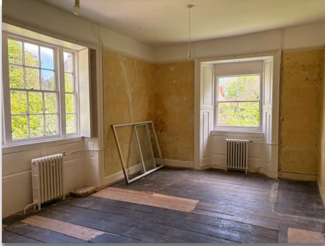
Figure 49. Bedroom 1. Note ad hoc timber replacement.
