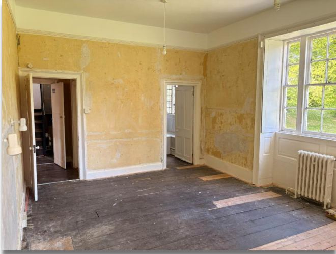
Figure 53. Bedroom 1; Wall between bedroom and ensuite.
