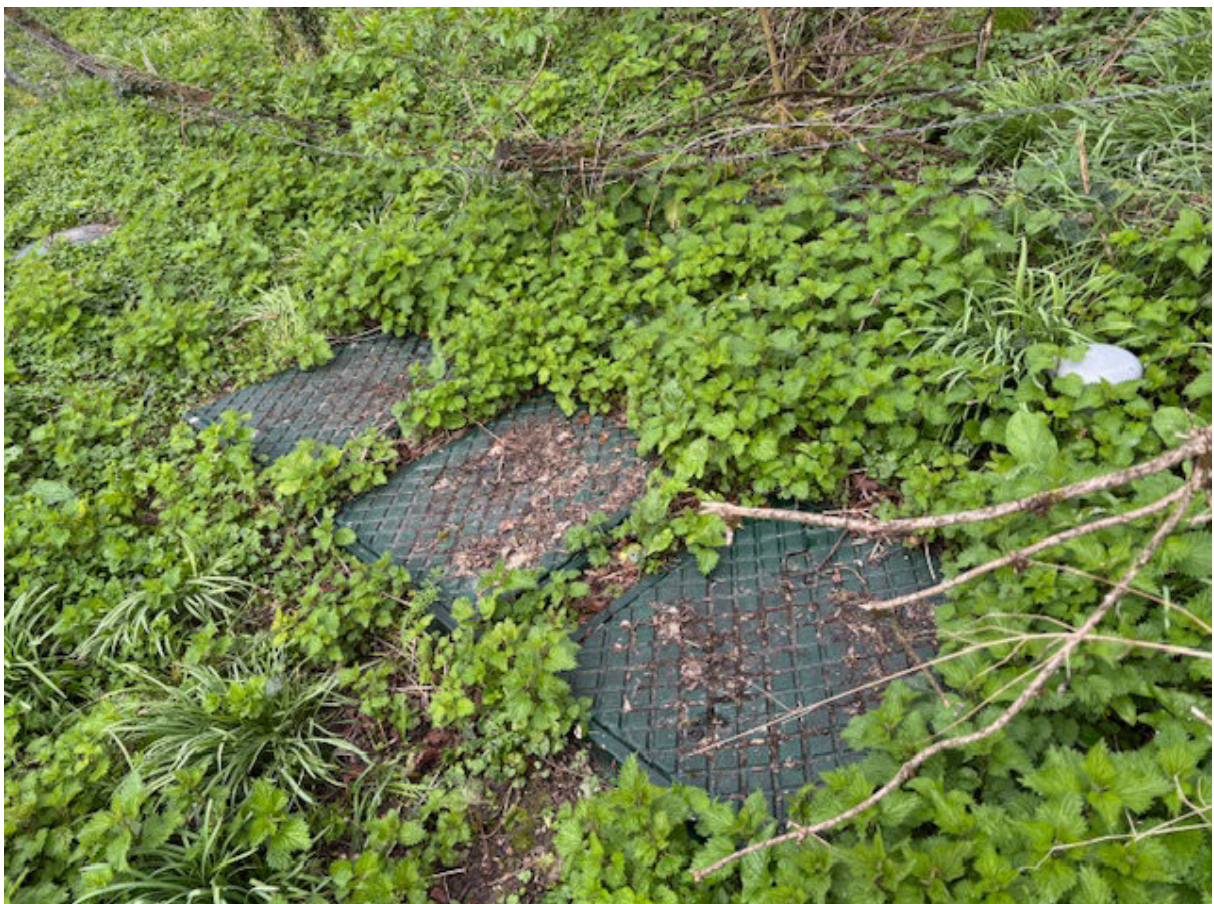
Photo 2: x3 entrance points to STP. Whilst not possible to open, the STP can be heard to be working.
