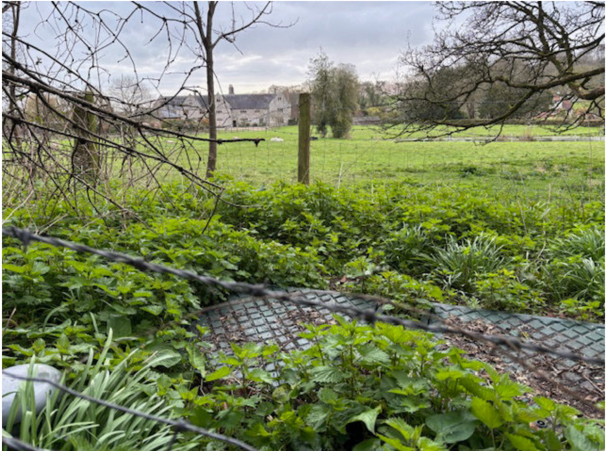
Photo 1: Existing 12 person STP showing the Manor House, Winterbourne Stoke that it serves, in the background
