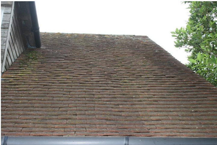
Photo 10: Lifted tiles on the annexe (B1).
