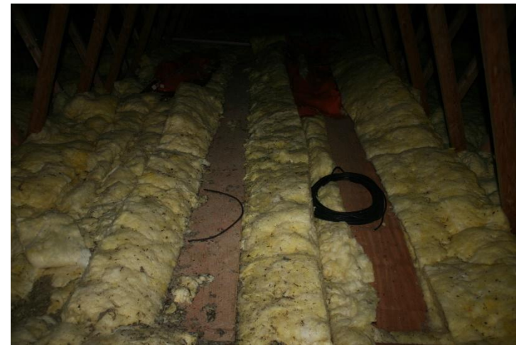
Photo 3: Bat droppings scattered in the loft.
