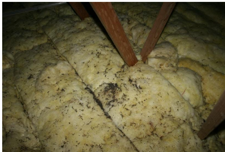
Photo 5: Bat droppings in the loft.
