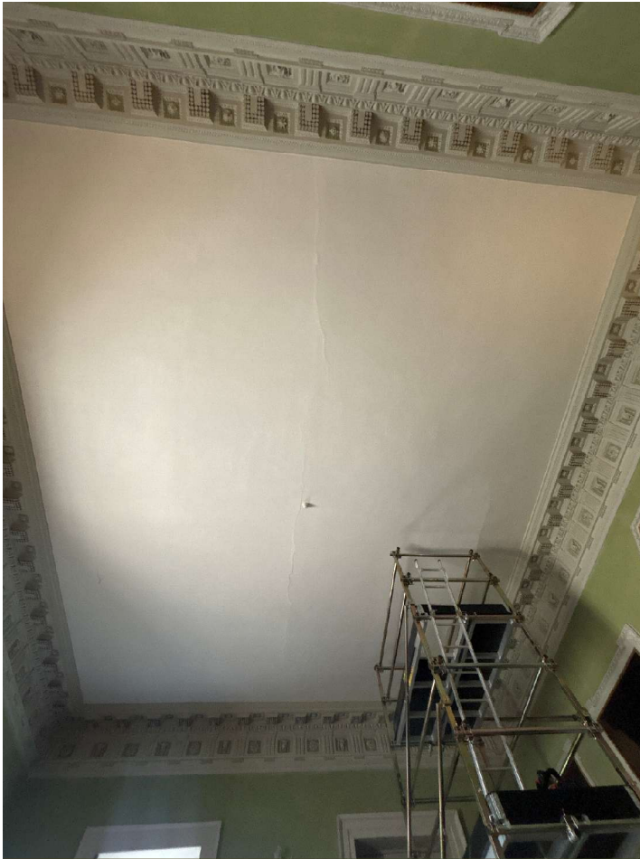
Dining room ceiling, with visible cracking along the midline. Worst cracking located above the scaffold tower position.
