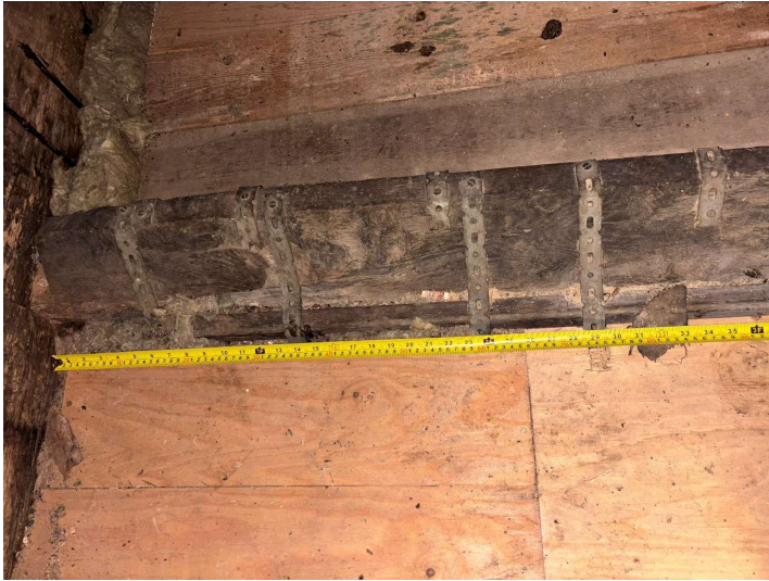
Historic strapping repair to failed secondary ceiling beam – see previous report for details.
