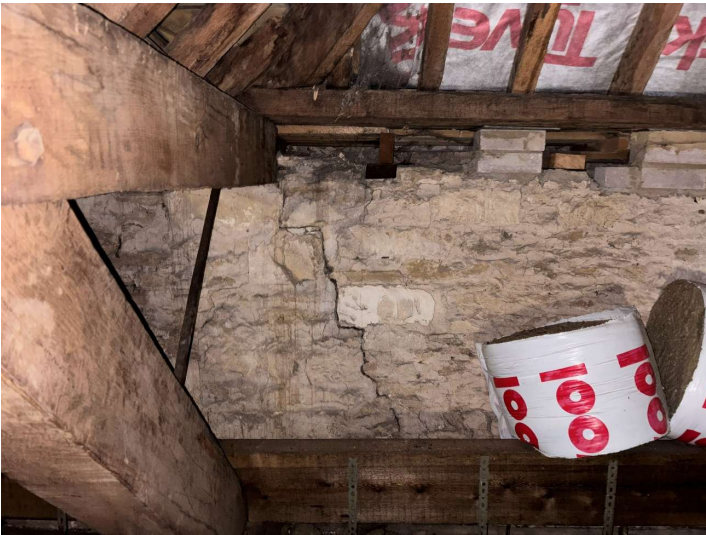
Northern wall with cracking beneath bearing of girder truss.
