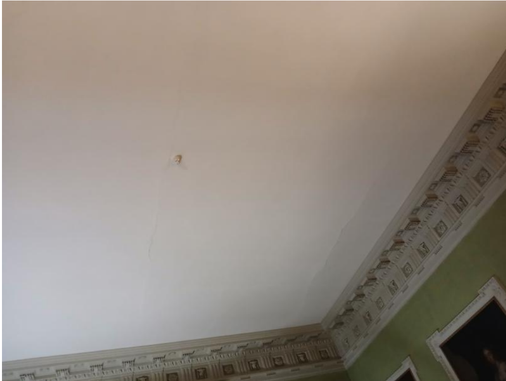
Figure 1 - Current cracks to dining room ceiling - looking towards northwest
