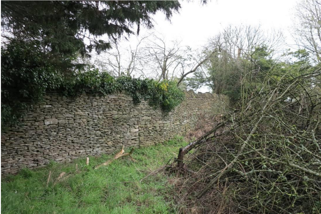
Plate 7. Boundary wall to the south-west of the listed converted barn; note the partial straight joints, which appear to describe an infilled opening but do not continue to the full height of the wall, suggesting the upper element has been rebuilt
