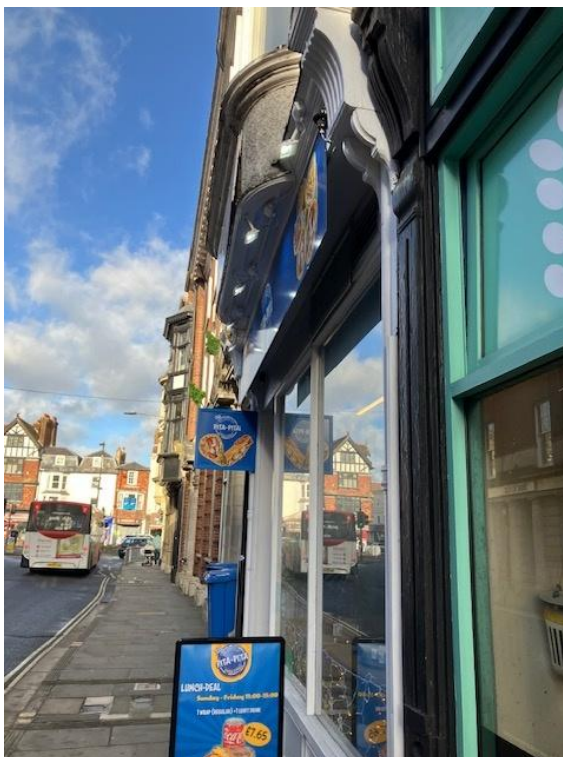
Unauthorised signage as existing
