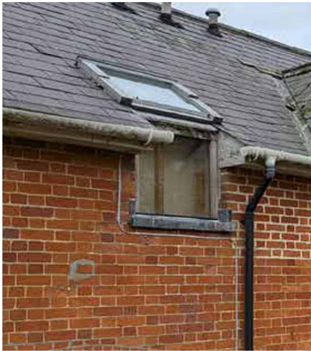
Existing over eaves window - in poor condition.
