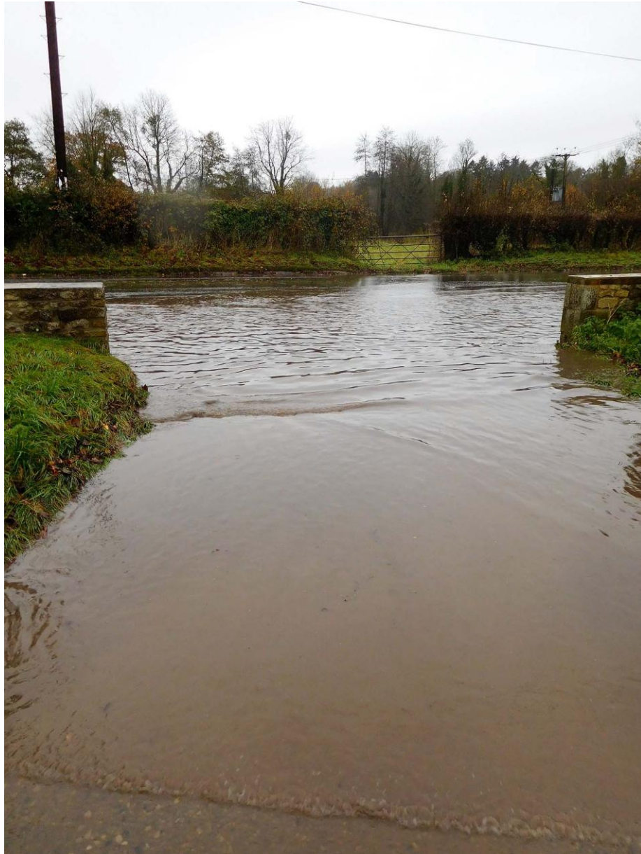
Flooding at Home Farm Lane entrance
