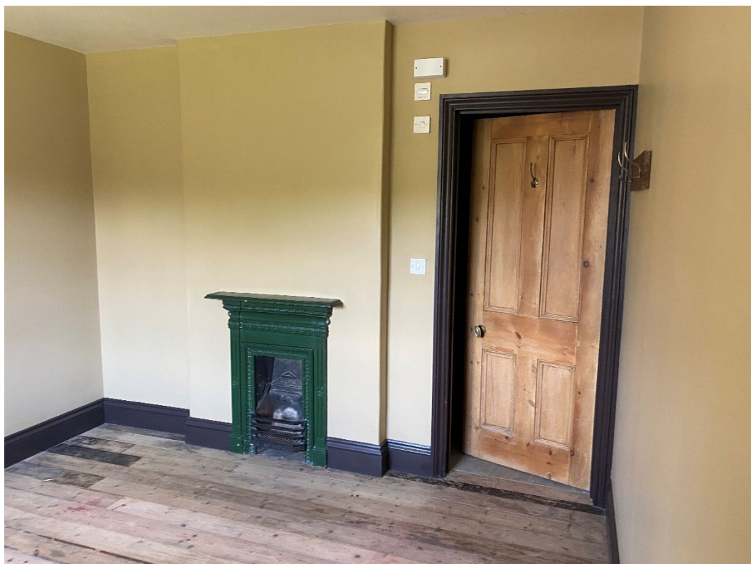
Figure 20: Ground floor room. Broadly appropriate Victorian grade and door style utilised in conversion.
