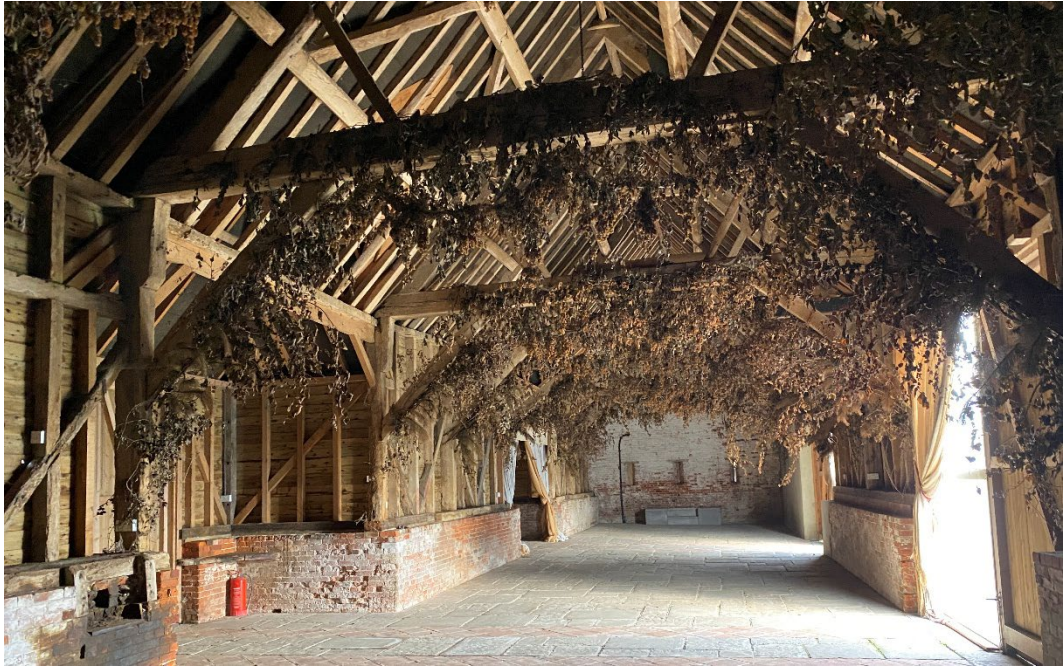
Figure 28: The barn, modern repairs and a floor but with strong historic architectural interest.
