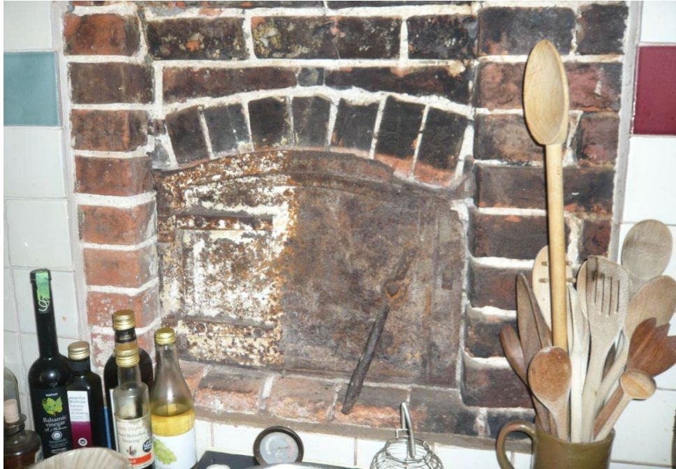
Figure 30: Former bread oven door as recorded in the 2014 Heritage Statement (Elain Milton Heritage and Planning, Figure 13, p.11) no longer present in the building.
