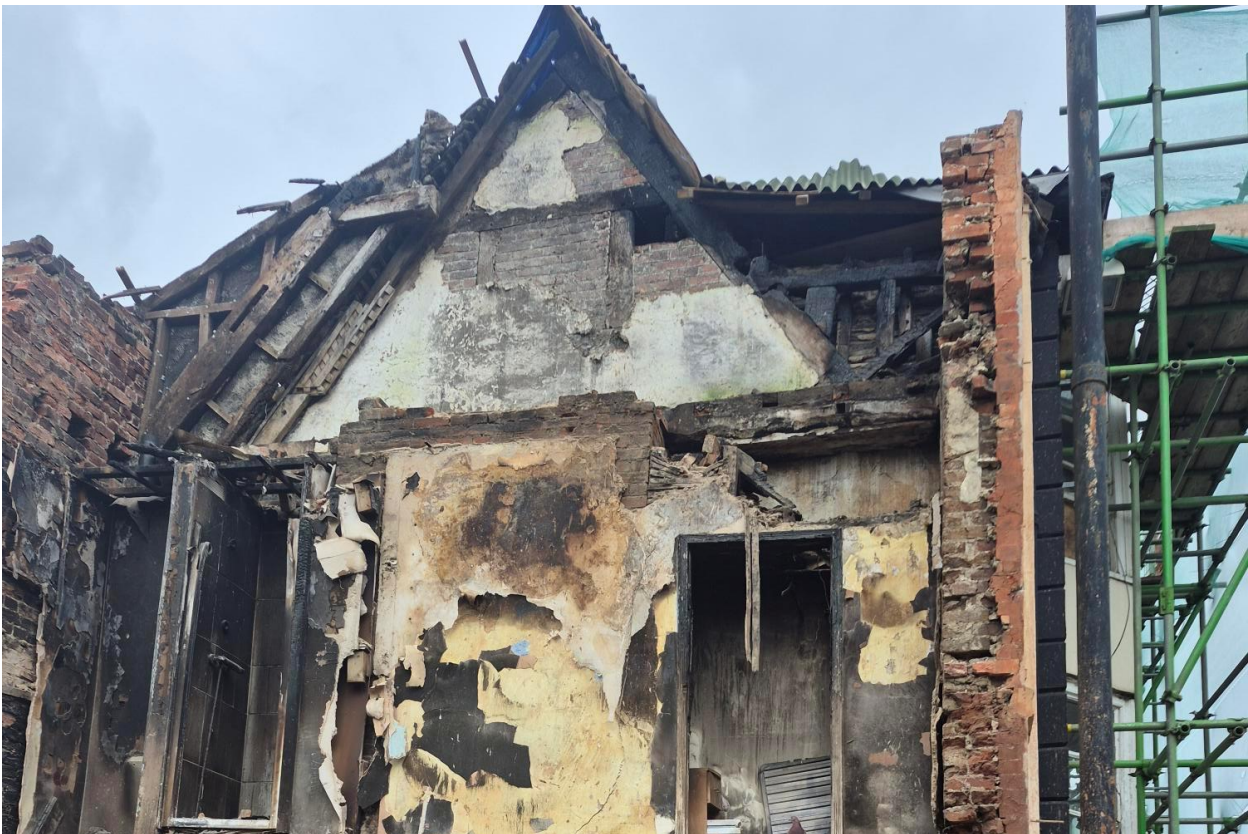
The fire damaged SE gable wall of No.3 Northgate Street following the demolition of No.2 Northgate Street.
