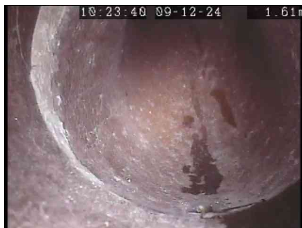
WCX_68817590-9c3b-4920-bbbe-ad50cd0abec5_20241211_125303_083.jpg, 00:00:22, 1.61 m Line of sewer deviates up, Rest bend
