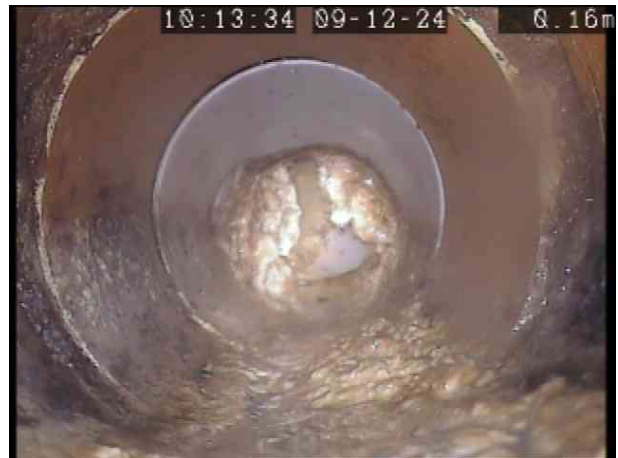
SVP1X_32eb4c9d-ff26-42db-ad52-19f29558d6cb_20241211_124323_505.jpg, 00:00:14, 0.16 m Debris, grease from 5 o'clock to 7 o'clock, 15% cross-sectional area loss
