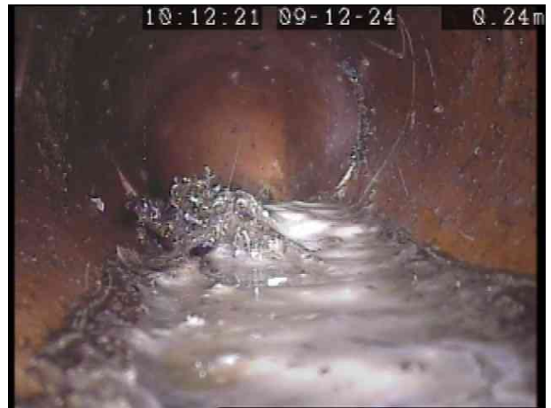
FG1X_a466e43c-4f62-41f8-84e2-a58d6ec7e930_20241211_1 24052_375.jpg, 00:00:40, 0.24 m Debris, other, 10% cross-sectional area loss, Sludge
