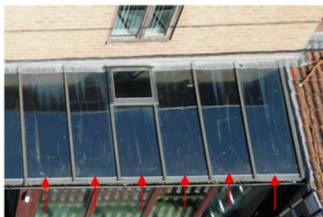
Image 10: Waiting Room External (Internal Cracked Panes).
