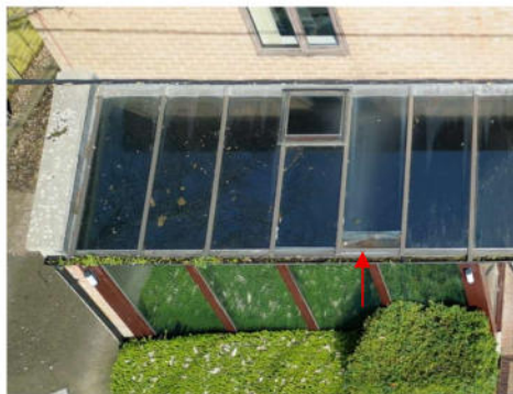
Image 8: Consultation Room External (External Cracked Pane).
