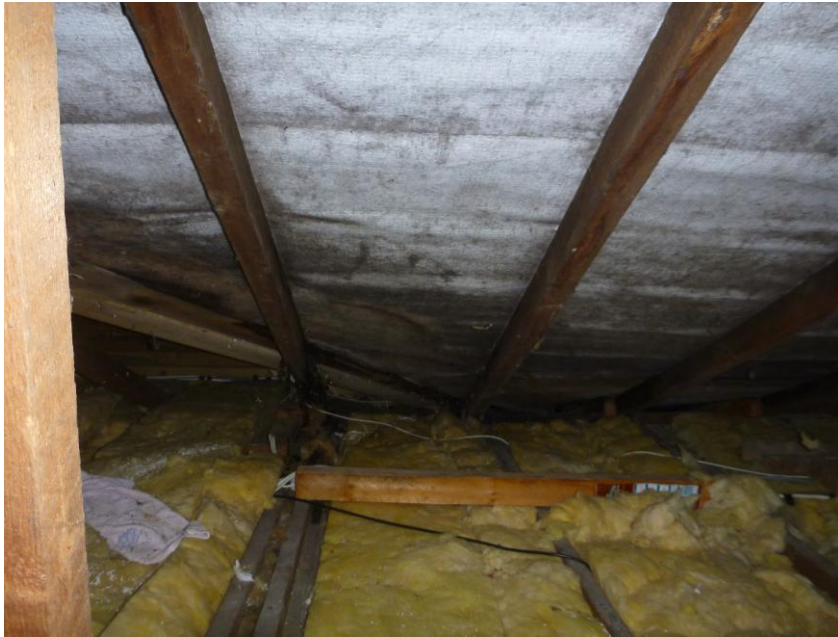
Fig 5: The property suffers from damp, which has caused some of the breathable membrane lining the roof to go mouldy.
